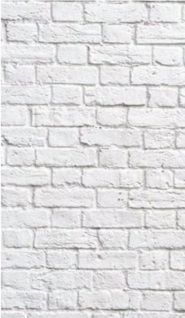
1 Existing Brickwork to be cleaned, existing white wash removed. Brickwork to be re-pointed where necessary and a new White Wash applied.
