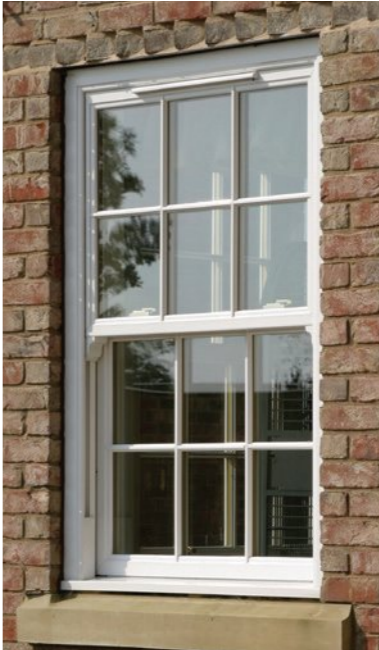
2 Replace removed and damaged windows with New Timber Sliding Sash with double glazing.
