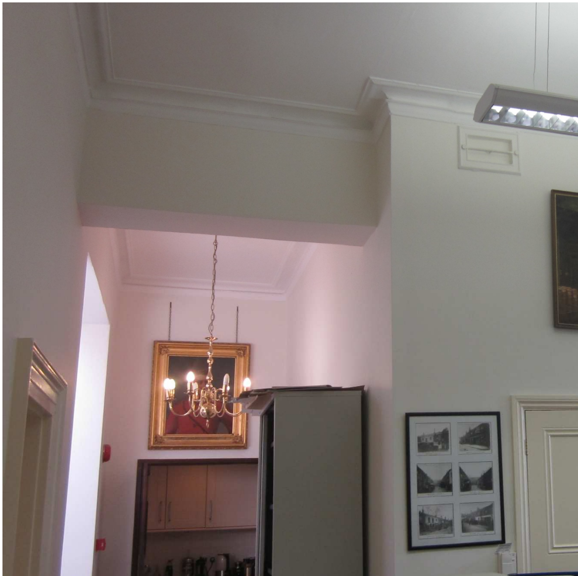
Photograph taken from RE.F02 looking towards existing kitchenette (RE.F07) with non-original wall dividing rooms RE.F01 & RE.F06 behind the filing cabinet on the right hand side.
