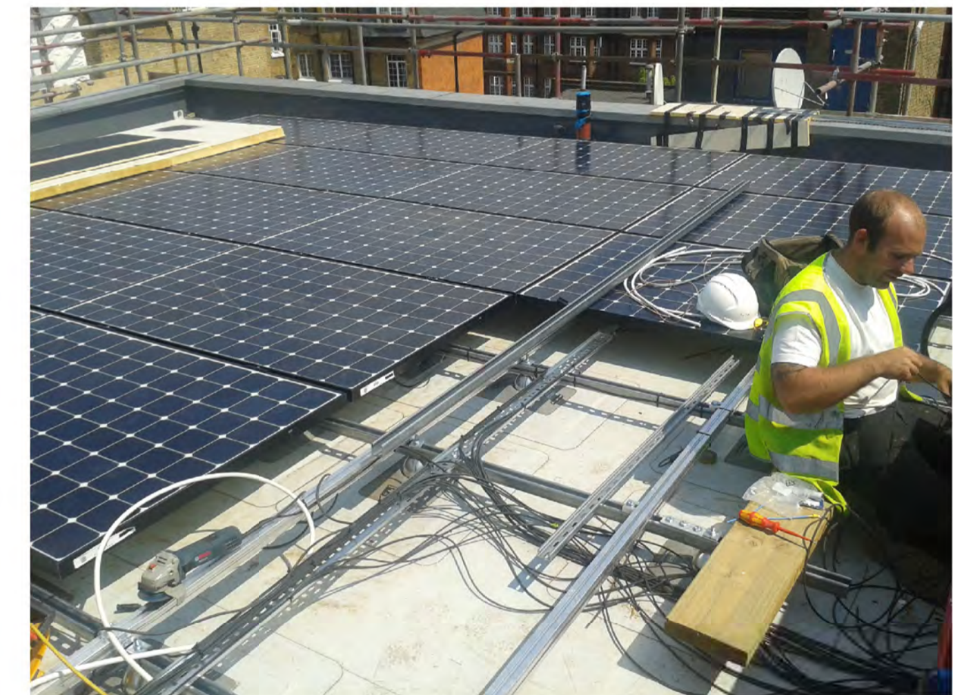
Image of installed PV panels
