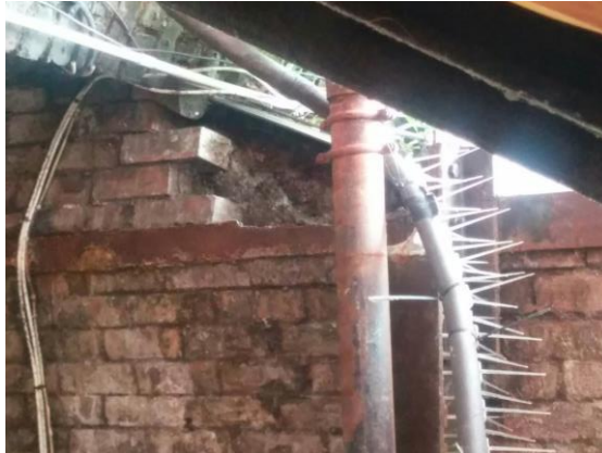
Figure 4: bricks missing from the walkway
