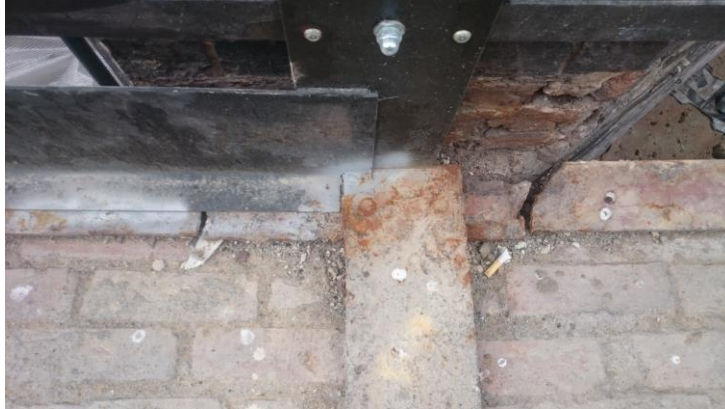
Figure 2: Secondary beams SB3-16 and SB3-17 showing poor structural condition
