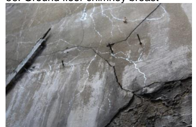
57. Ground floor cracked render
