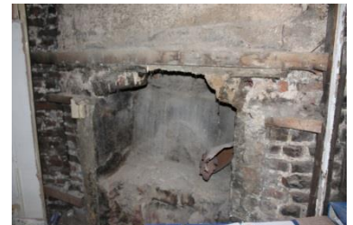
19. Rear chimney breast to be repaired
