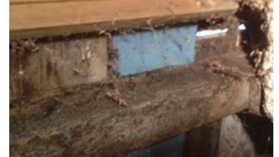
28. Rotten beam supporting shop front
