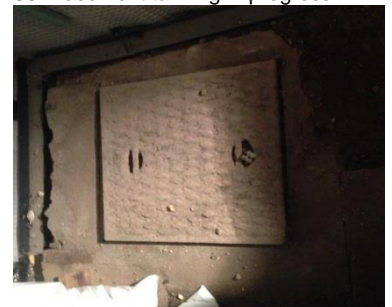
37. Vault manhole cover to be renewed With a double sealed cover to comply with current standards
