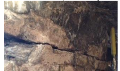
31. Cracked brickwork beneath shop front
