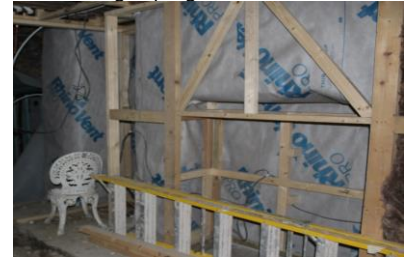
34. Dry lining in front of tanking in progress, front fireplace encased in dry lining. No structural alterations have been made and this work is reversible
