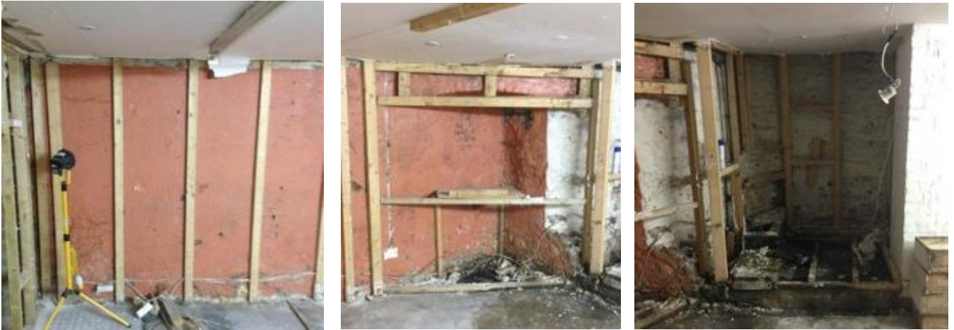
69-71. Basement rear dry lining in progress and ceiling renewed with a void for service routes (photos by Debby Lee during opening up after removal of plasterboard linings)
