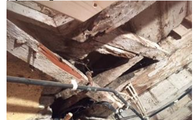
46. Joists at rear of basement replacement to be to engineer's details
