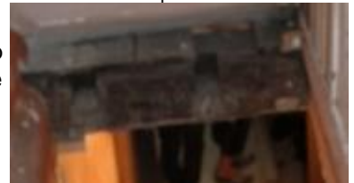
66. Close-up of trimmer to be relocated, showing notches for original joist ends so to be re-used as it shows the history
