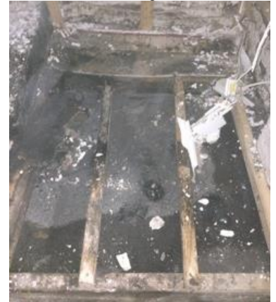
45. Basement rear floor after removal of ply casing – no historic floors remain
