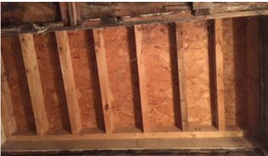
53. Existing infilled opening to be adapted with trimmers and re-used for roof-light
