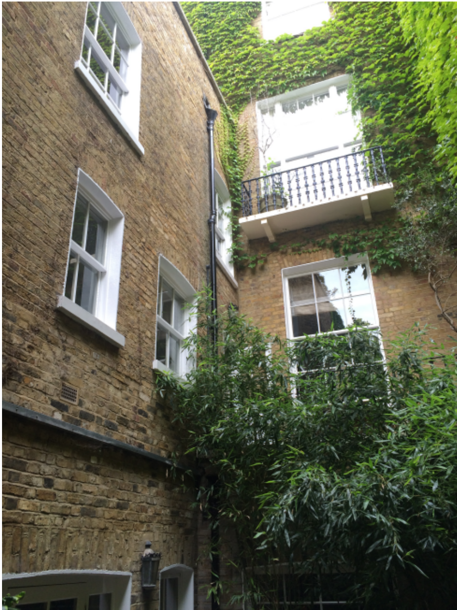
7. Looking at the rear wall of the main house and side wall of the infill extension
