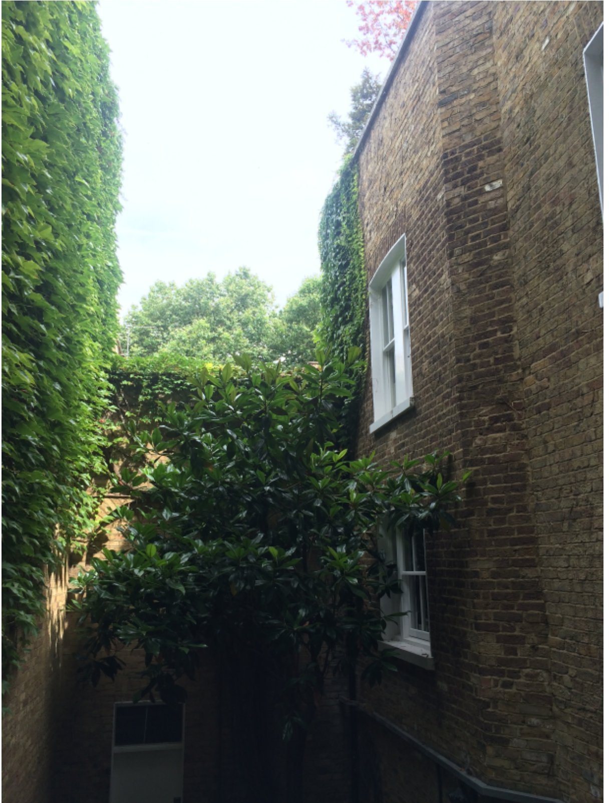
8. View from the first floor – arches on the rear of the mews behind the tree.
