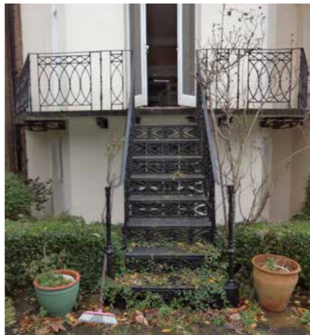
Rear balcony to Ground Floor Reception room; canted bay with stone plinth, cast iron support to stone plinth, wrought iron balustrade, cast iron staircase, and cast iron balusters to staircase
