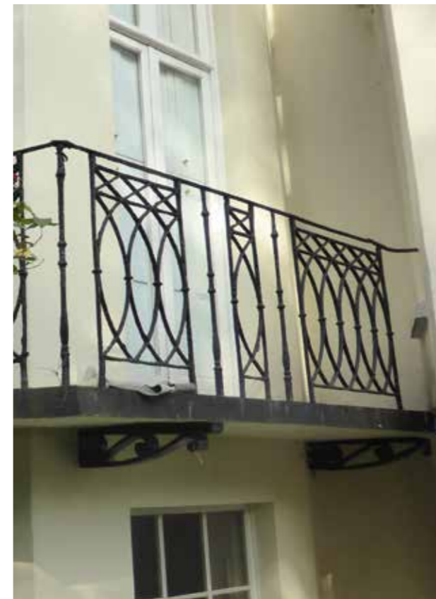
Existing cast iron support to stone plinth, detail to be retained and repaired
