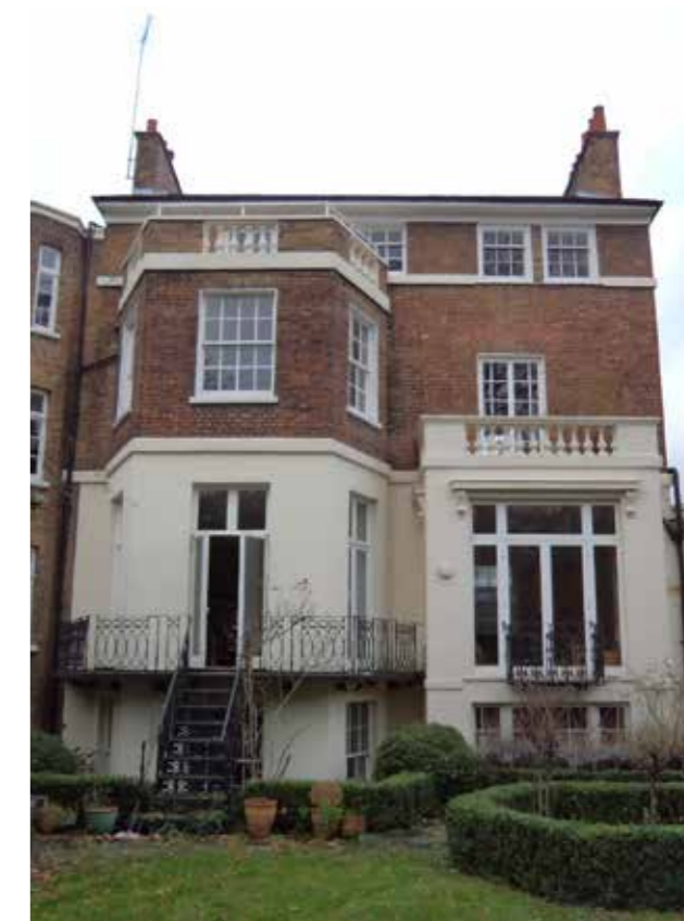
Existing window WSF-05, just visible at top right corner of bay, proposed to be realigned
