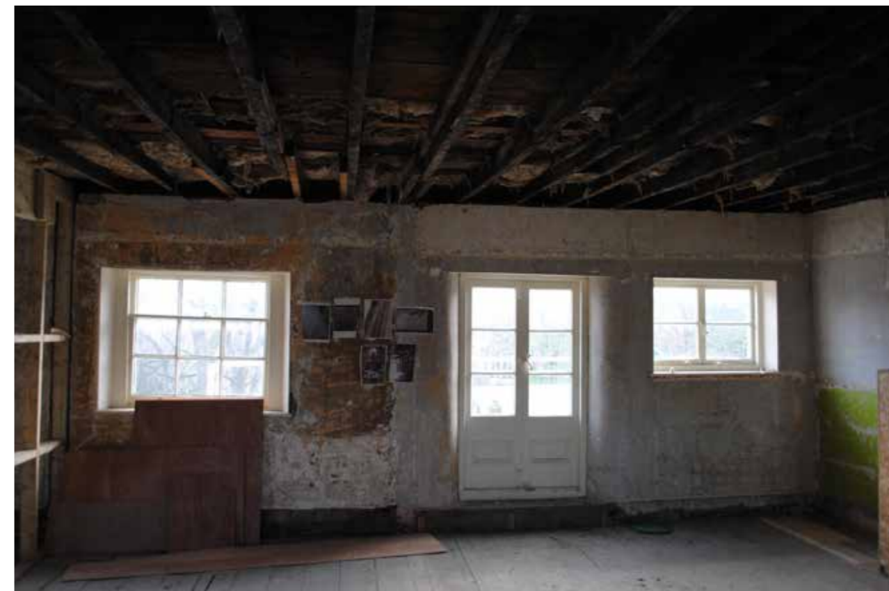
Existing window WSF-05 (left) & WSF-04 (right), proposed to be realigned to balance with each other, and be centred around the terrace door
