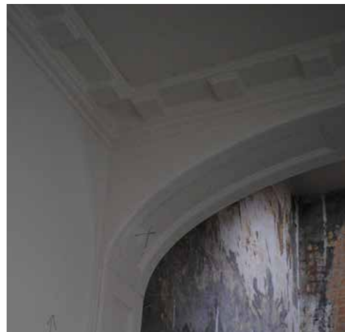
Ceiling moulding to cornice and architrave to arch in hallway to remain
