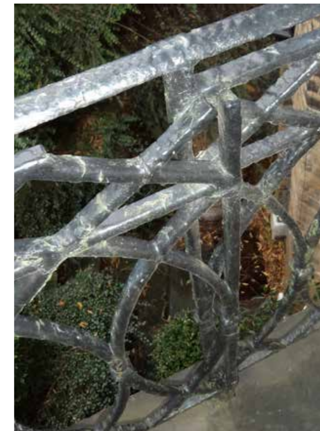
Existing wrought iron detail to canted bay, detail to be retained and repaired
