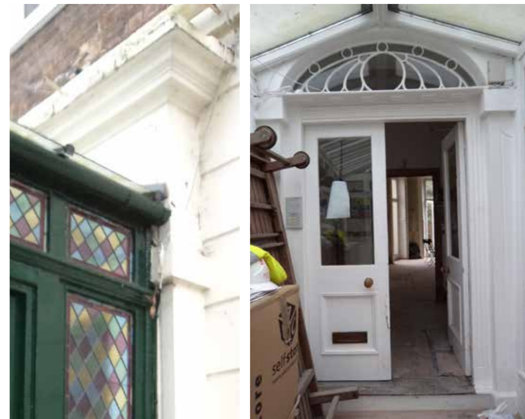
Existing Porch does not respectfully meet existing door surround and fanlight
