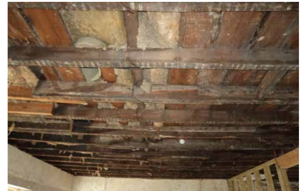
First Floor missing ceiling
