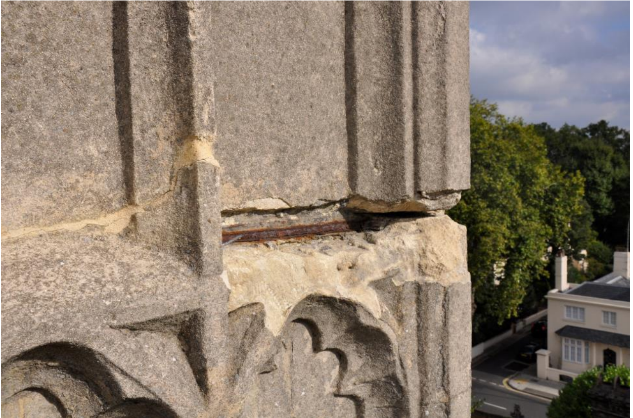
Photo 03 – north tower, spalled stonework and repairs revealing assumed wrought iron band behind
