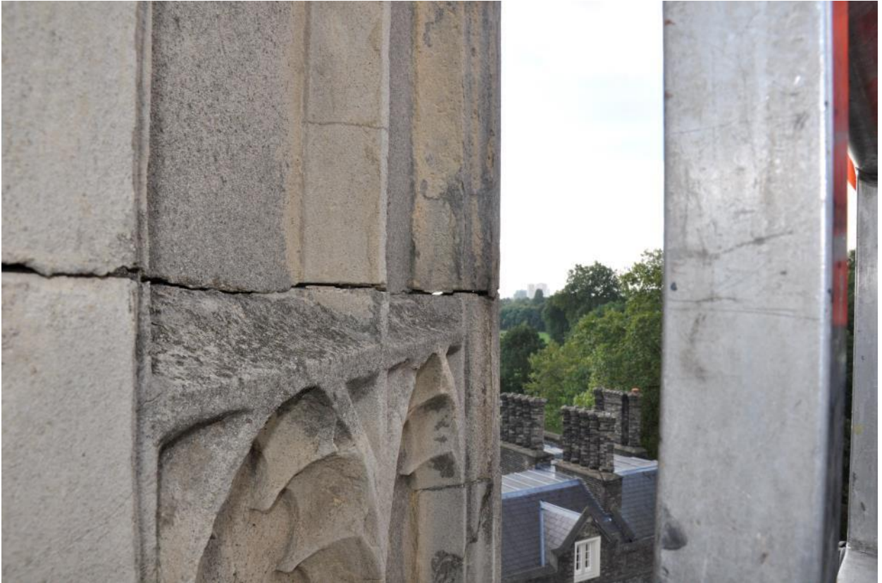
Photo 05 – south tower, parting in bed joint between traceries (level or wrought iron band)
