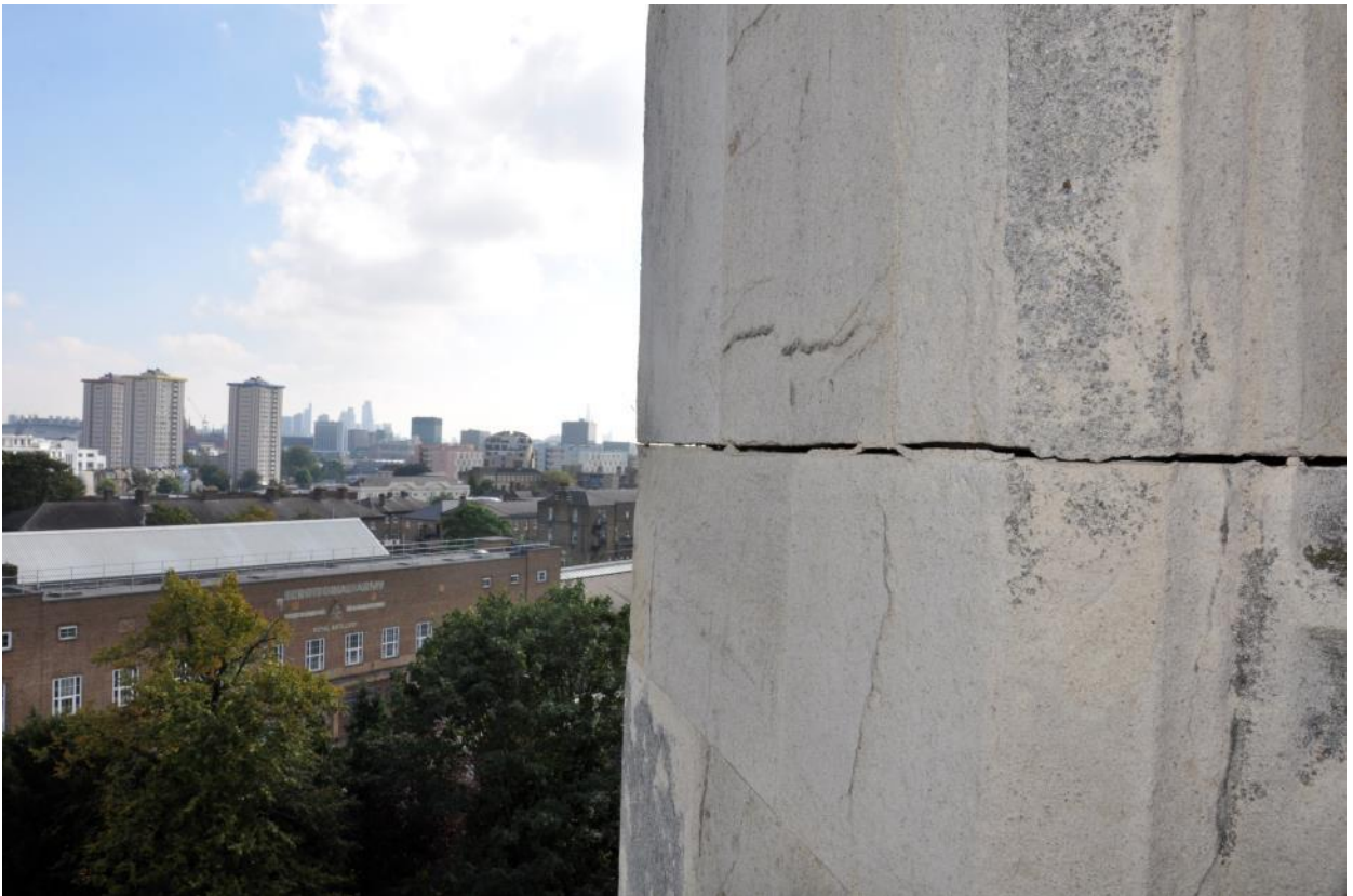
Photo 06 – south tower, parting in bed joint along non-decorated face (level or wrought iron band)
