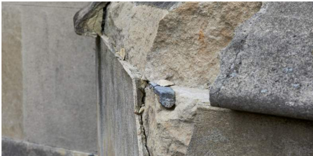
Fig 6. A detail view of the failing stone and rusting cramps (ABA)
