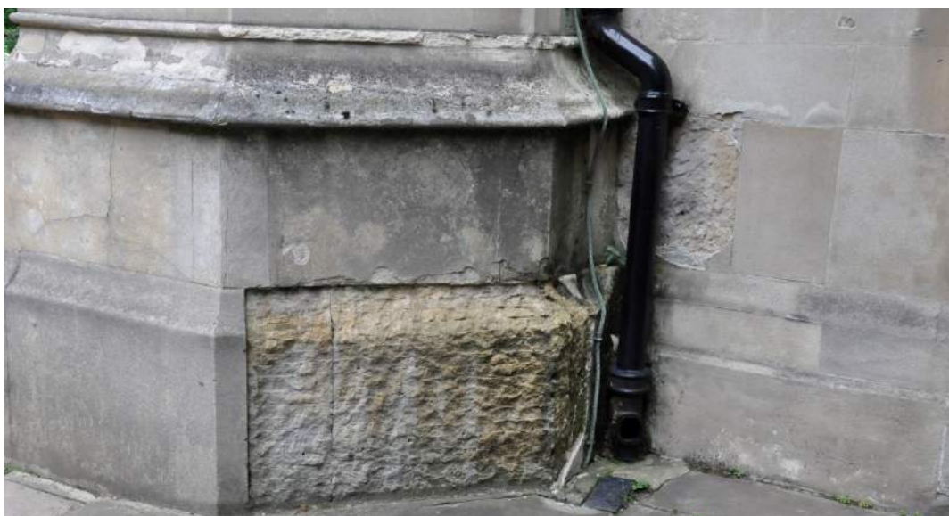
Fig 7. A view of the footings with decayed surface stone (ABA)
