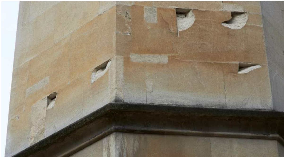
Fig 5. A view of the stone failure on the west end due to rusting cramps (ABA)
