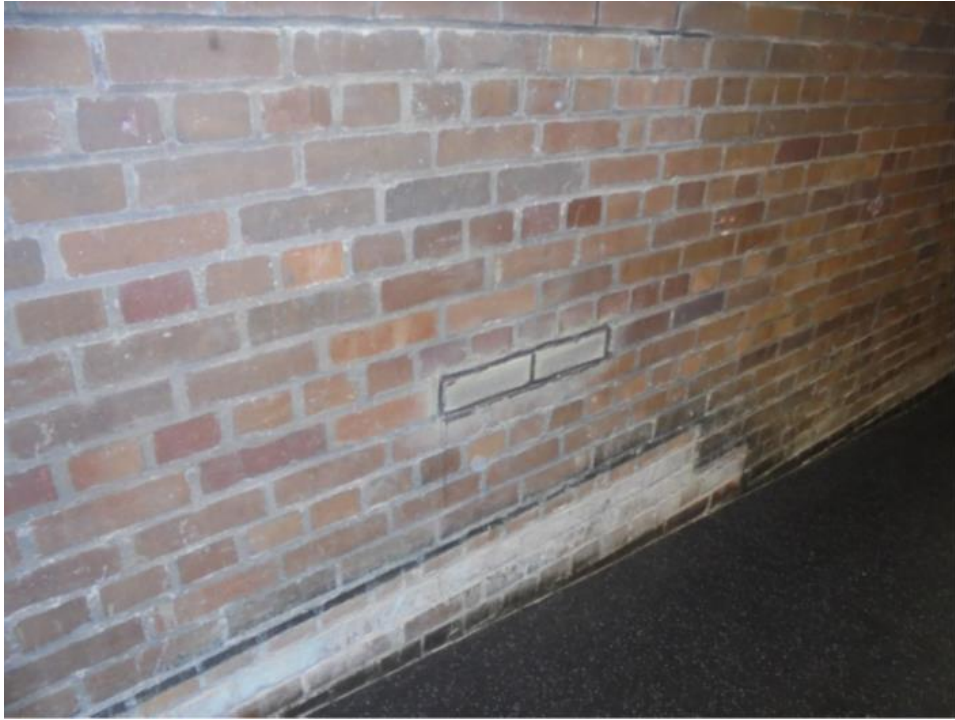
Poorly replaced bricks on the first floor of the link bridge
