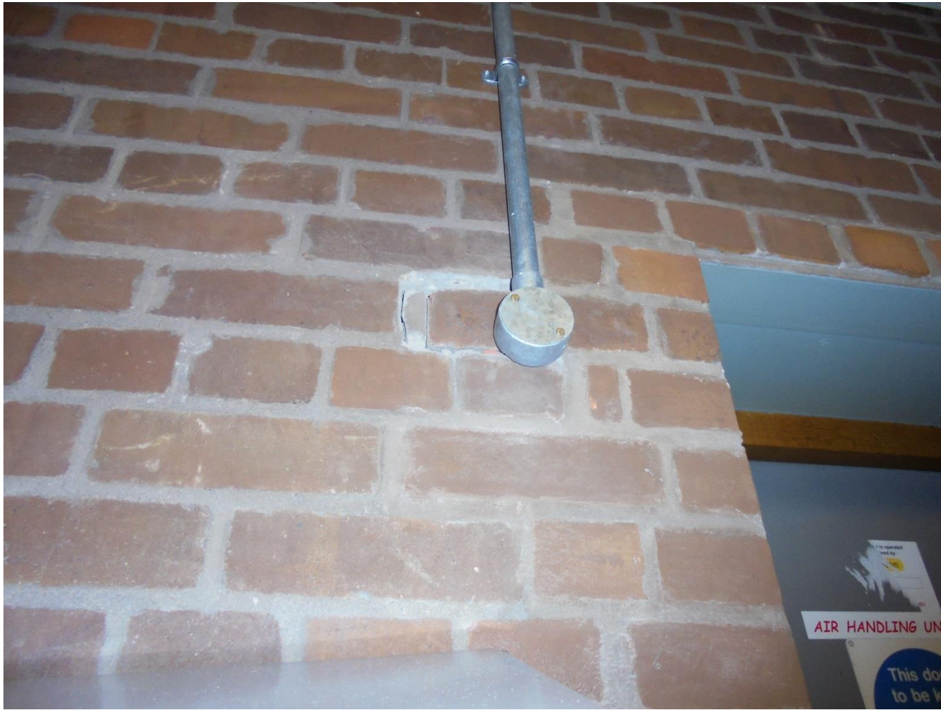
Internal face of cladding to the Link Bridge – proposed investigation through previously removed brick – Level 2 – location for works refs 3.2.1 & 3.2.2
