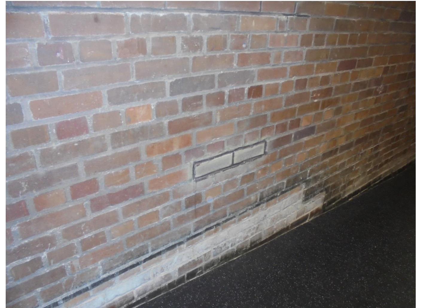
Internal face of cladding to the Link Bridge – proposed investigation through previously removed bricks – Level I – location for works refs 3.2.1 & 3.2.2
