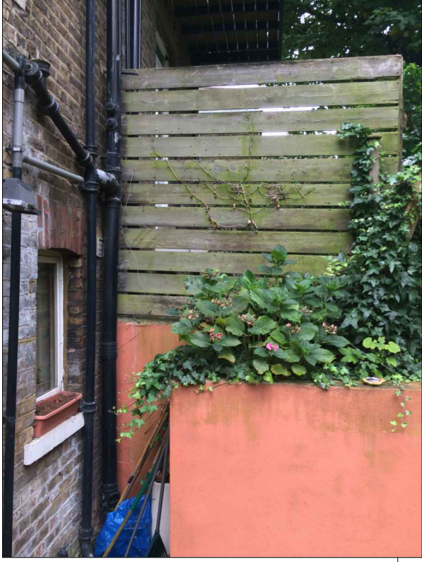
EXISTING MASONRY AND TIMBER GARDEN WALL ON A BOUNDARY WITH NO 27 KINGDON ROAD, APPROX HEIGHT 3.6M
