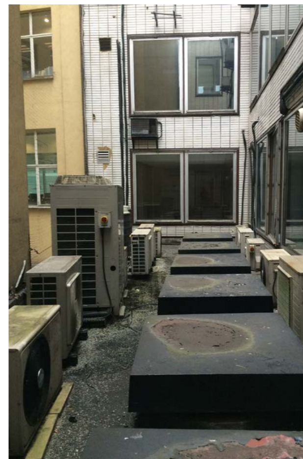
Visible plant equipment to 1st floor roof within lightwell
