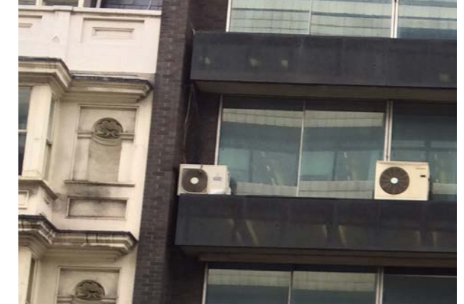
Visible external plant equipment on High Holborn facade
