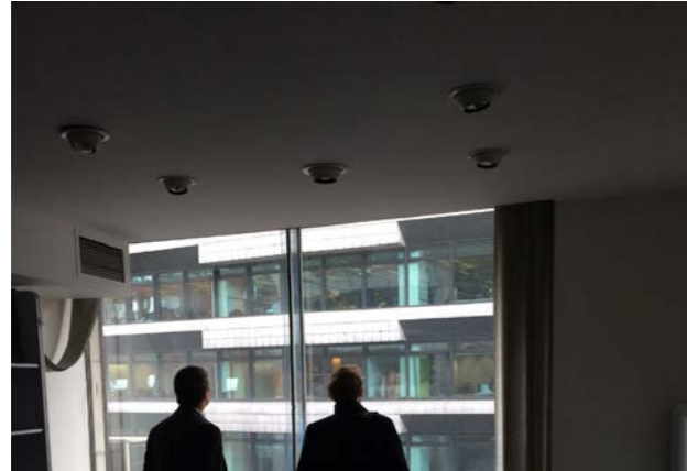
Typical chambers office space. Dropped bulkheads for heating and ventilation
