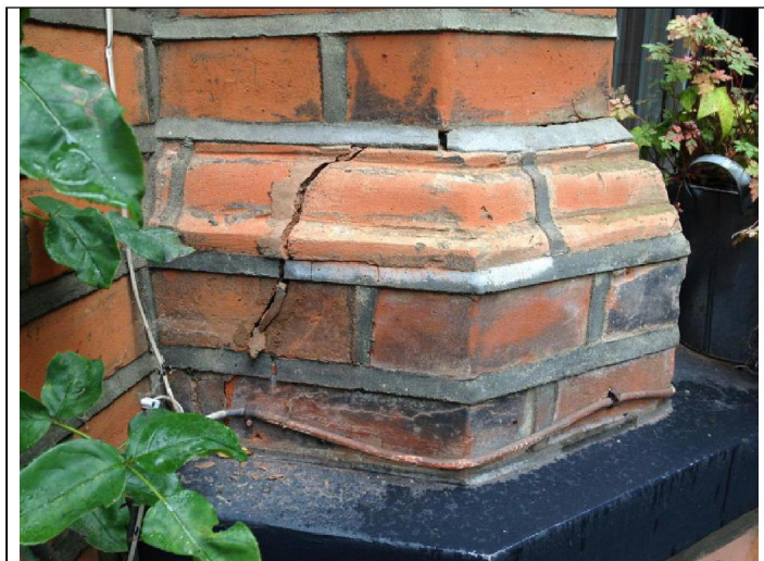
Cracking to pier of bay
