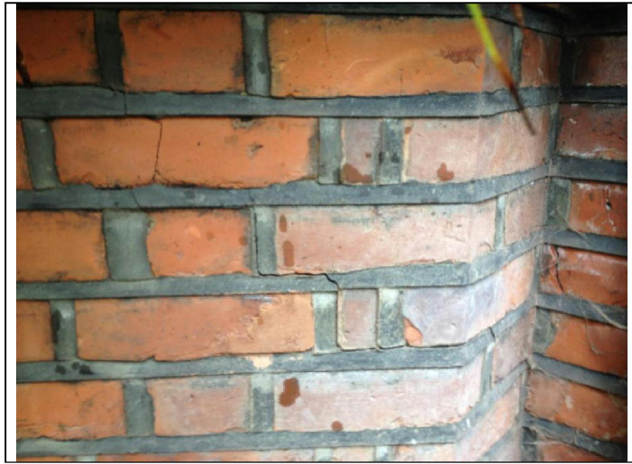
Cracking to bay
