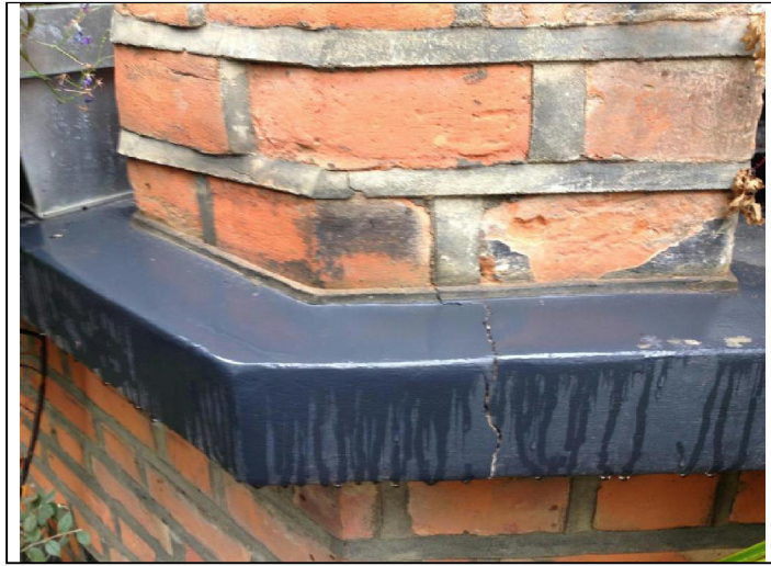
Cracking to sill of bay
