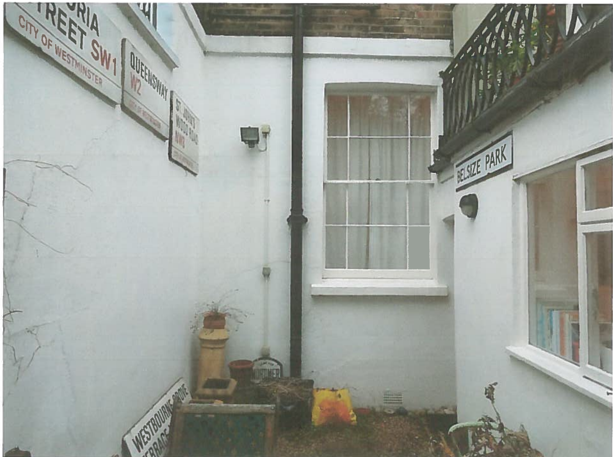
Photograph of the rear elevation at ground floor level - Kitchen window to the right and bedroom window facing.
