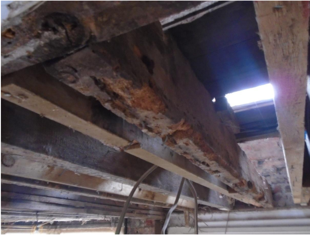
Image 25: Image of rotten joist
