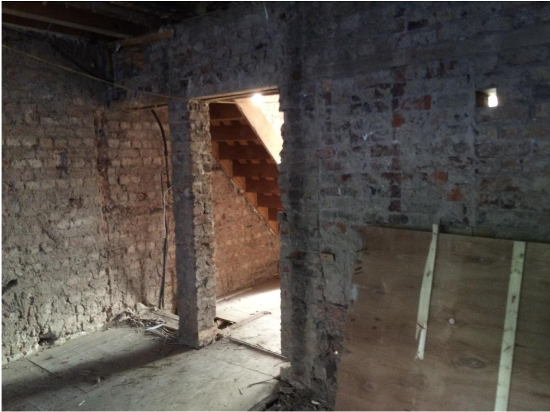
Image 14: Internal brick wall at lower ground floor, brick wall and pier in poor condition
