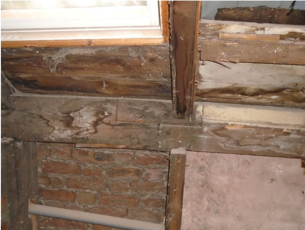
Image 30: Inadequate halving joint configuration and evidence of rot in roof waling beam
