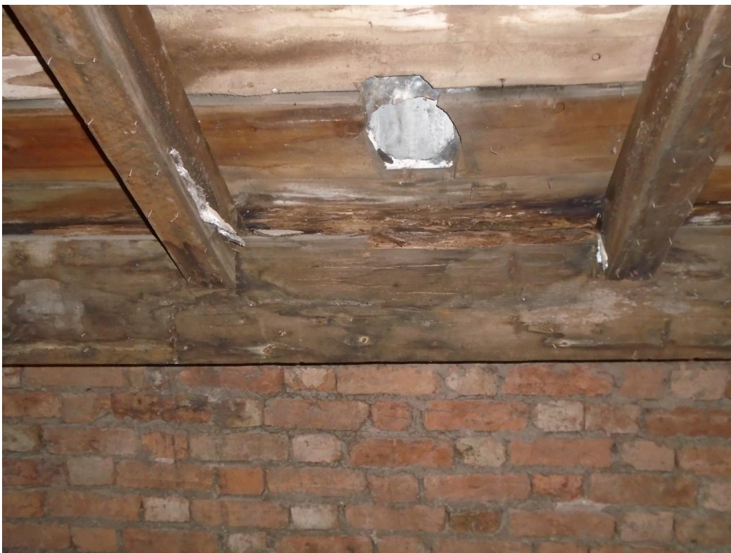
Image 28: Roof waling beam and rafter ends showing signs of rot – Image 2
