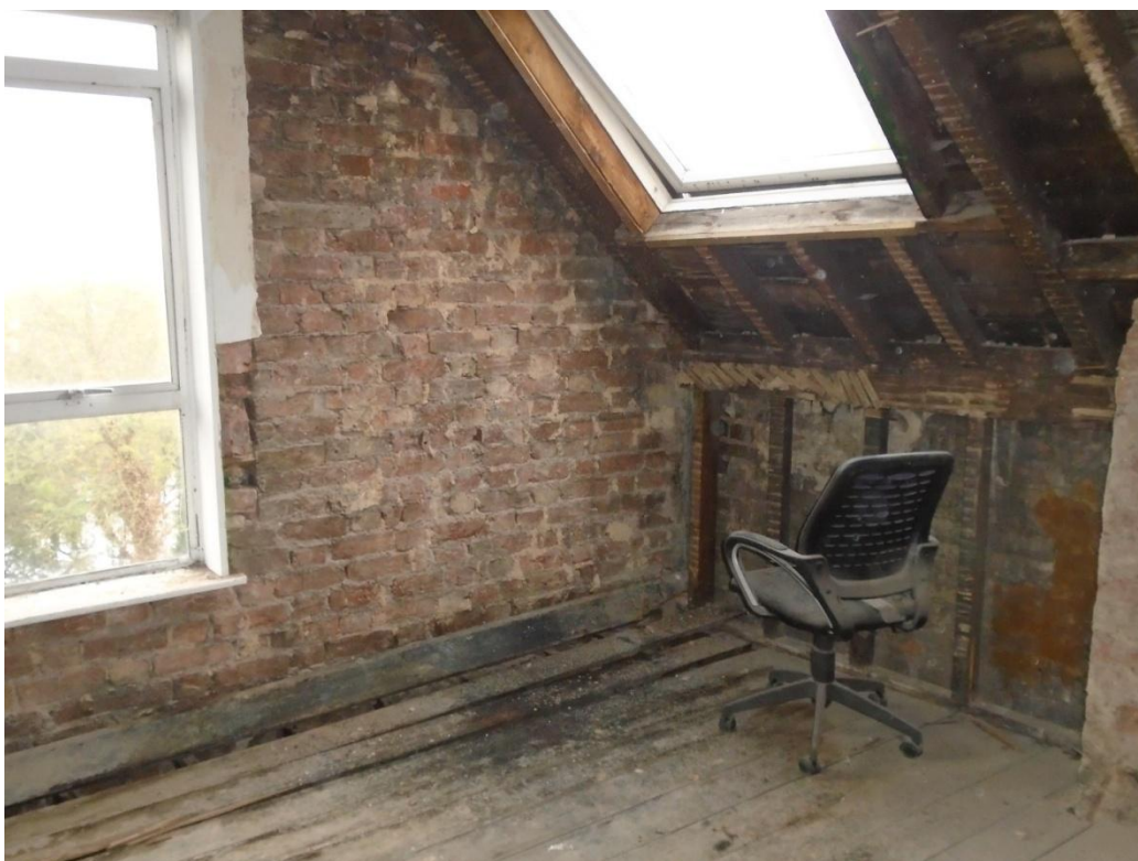
Image 39: Image of poor condition of brickwork and roof structure to rear facade
