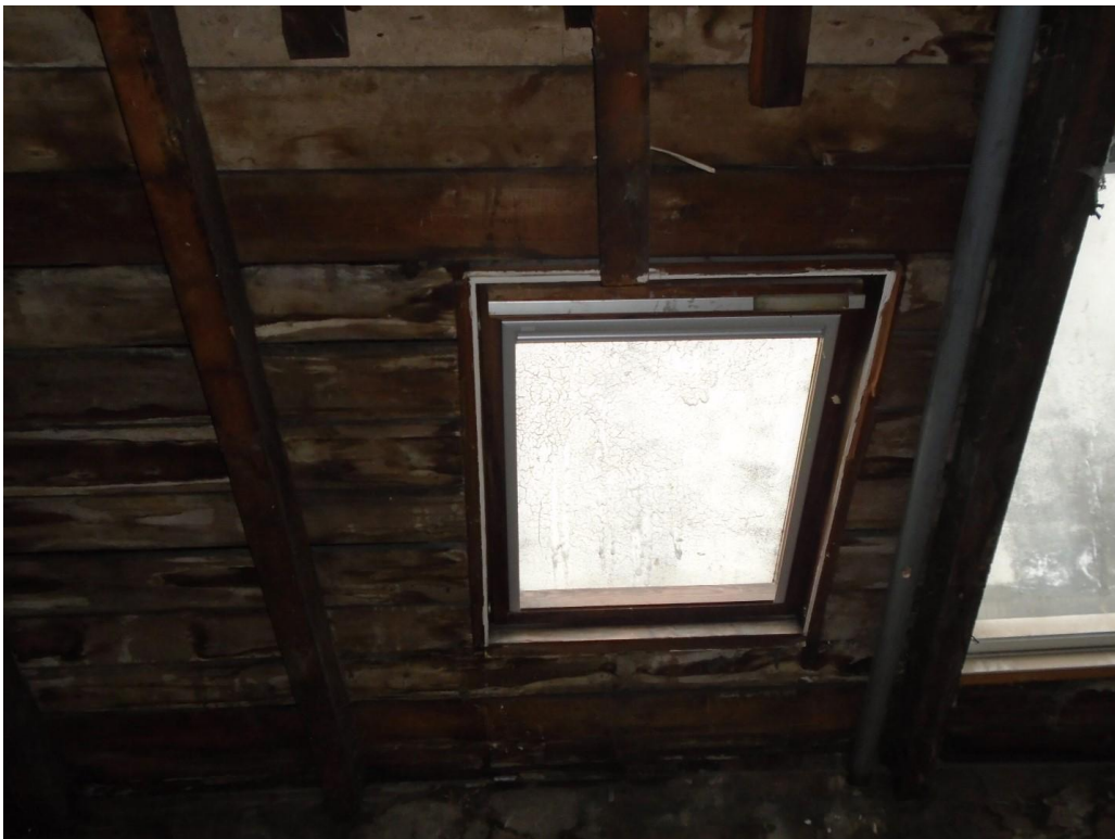
Image 35: Inadequate trimming to rafters around roof lights
