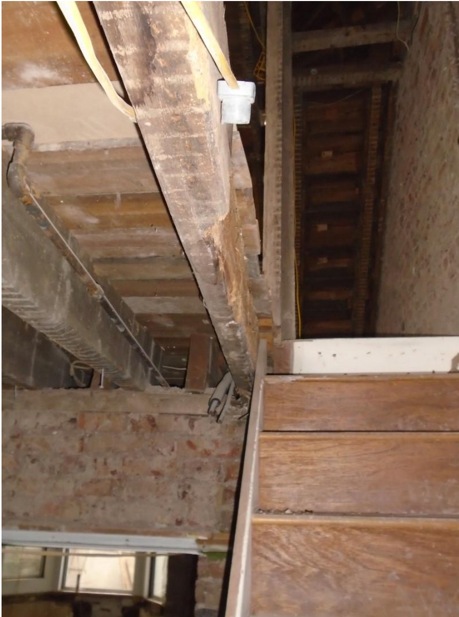
Image 18: Excessive notching of trimmer joist to stair void – Image 1
