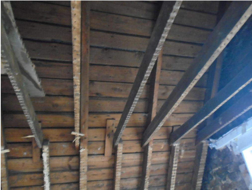
Image 32: Every second roof rafter has been cut at collar tie position over full length of roof rendering the roof structure inadequate and potentially dangerous
