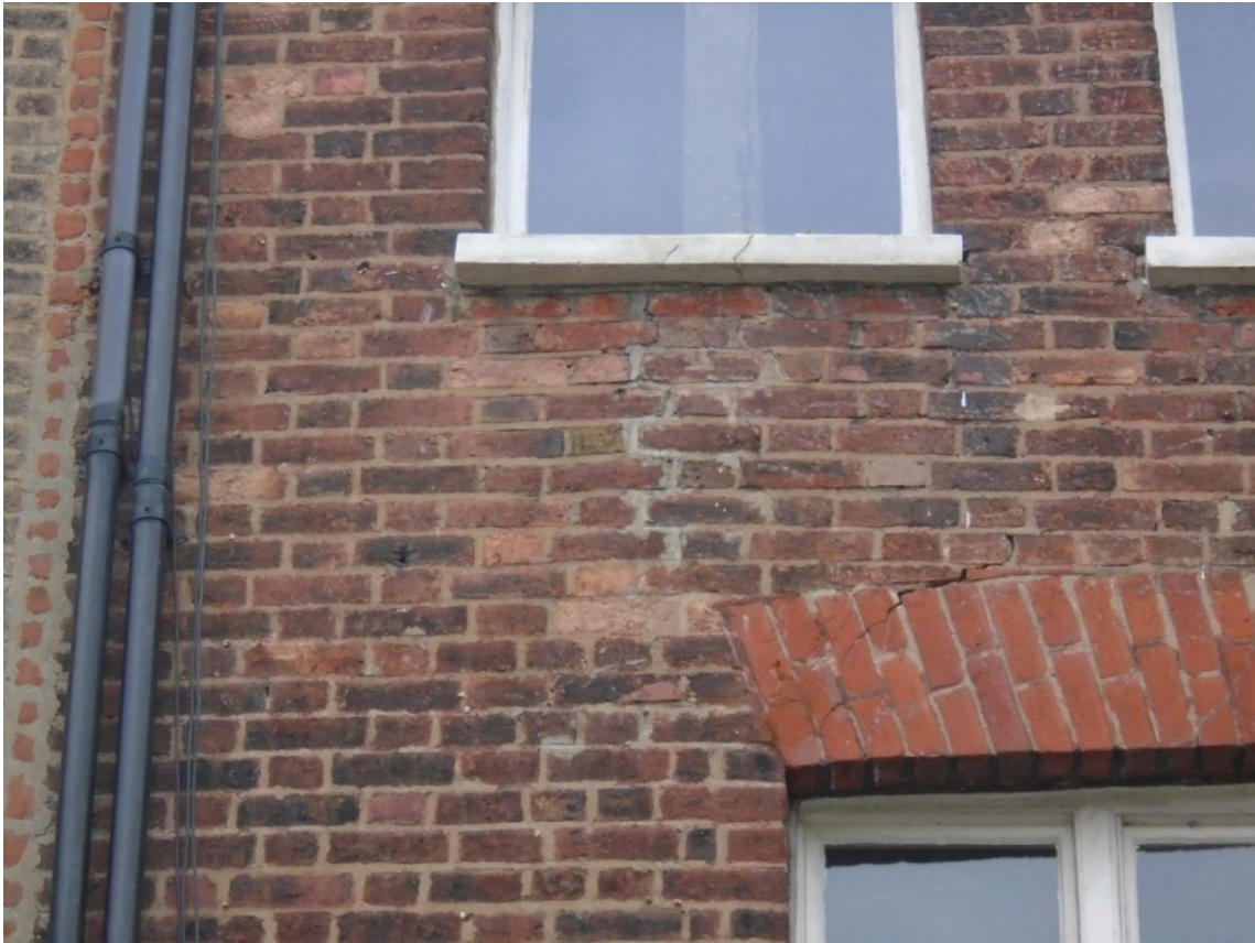
Image 2: Cracked lintel and exfoliation of brickwork to rear facade
