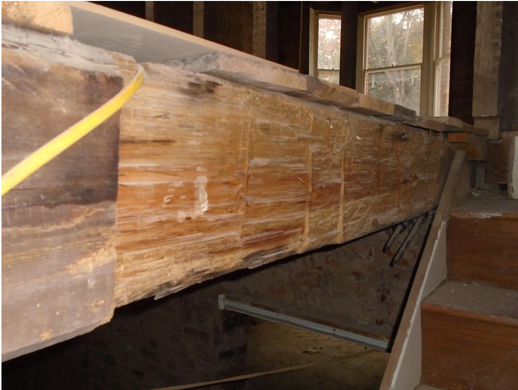
Image 19: Excessive notching of trimmer joist to stair void – Image 2
