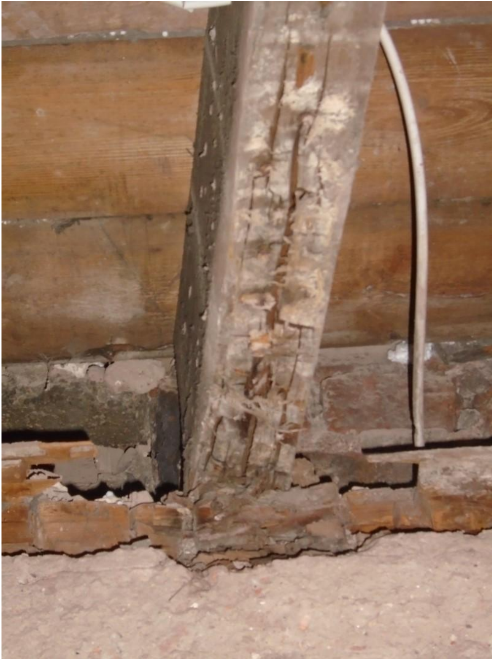
Image 11: Image of rotten floor joist
