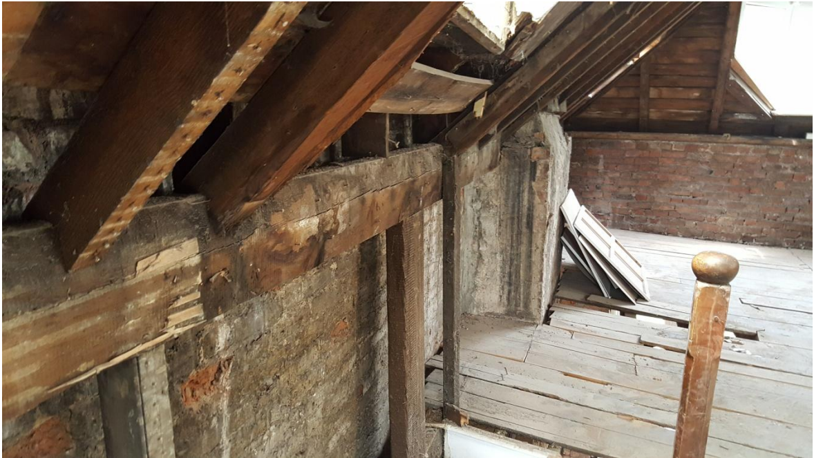
Image 41: Rotten waling timber supporting roof joists. Also timber studs supported from undersized floor joists. Generally substandard roof construction is evident throughout
