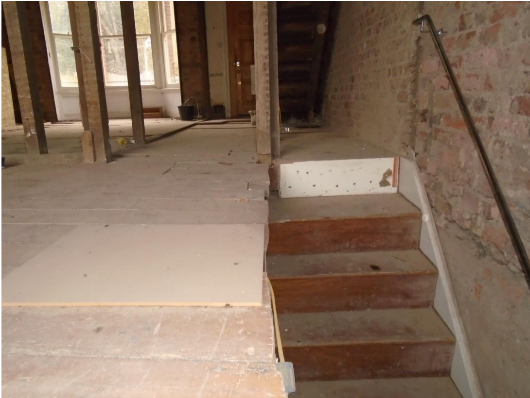
Image 21: Image showing excessive deflection of floor adjacent to stair void
