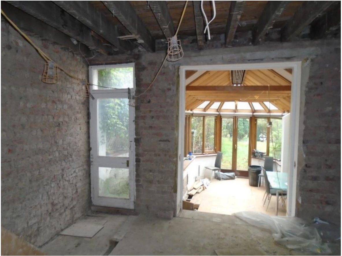
Image 6: Internal view of rear elevation showing excessive deflection of floor adjacent to rear door
