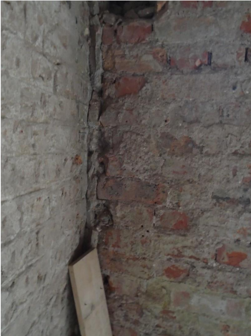
Image 8: Internal view of rear facade inadequately toothed in/tied to party wall – Image 2
