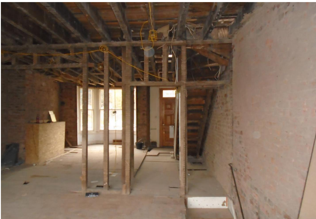
Image 20: Load-bearing stud (spine wall on upper floors) in poor condition and is structurally inadequate
