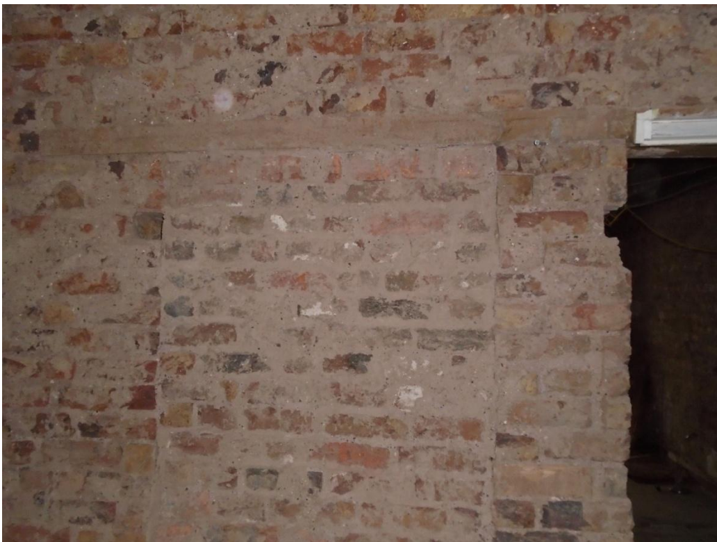
Image 17: Opening bricked up and brickwork not toothed in properly
