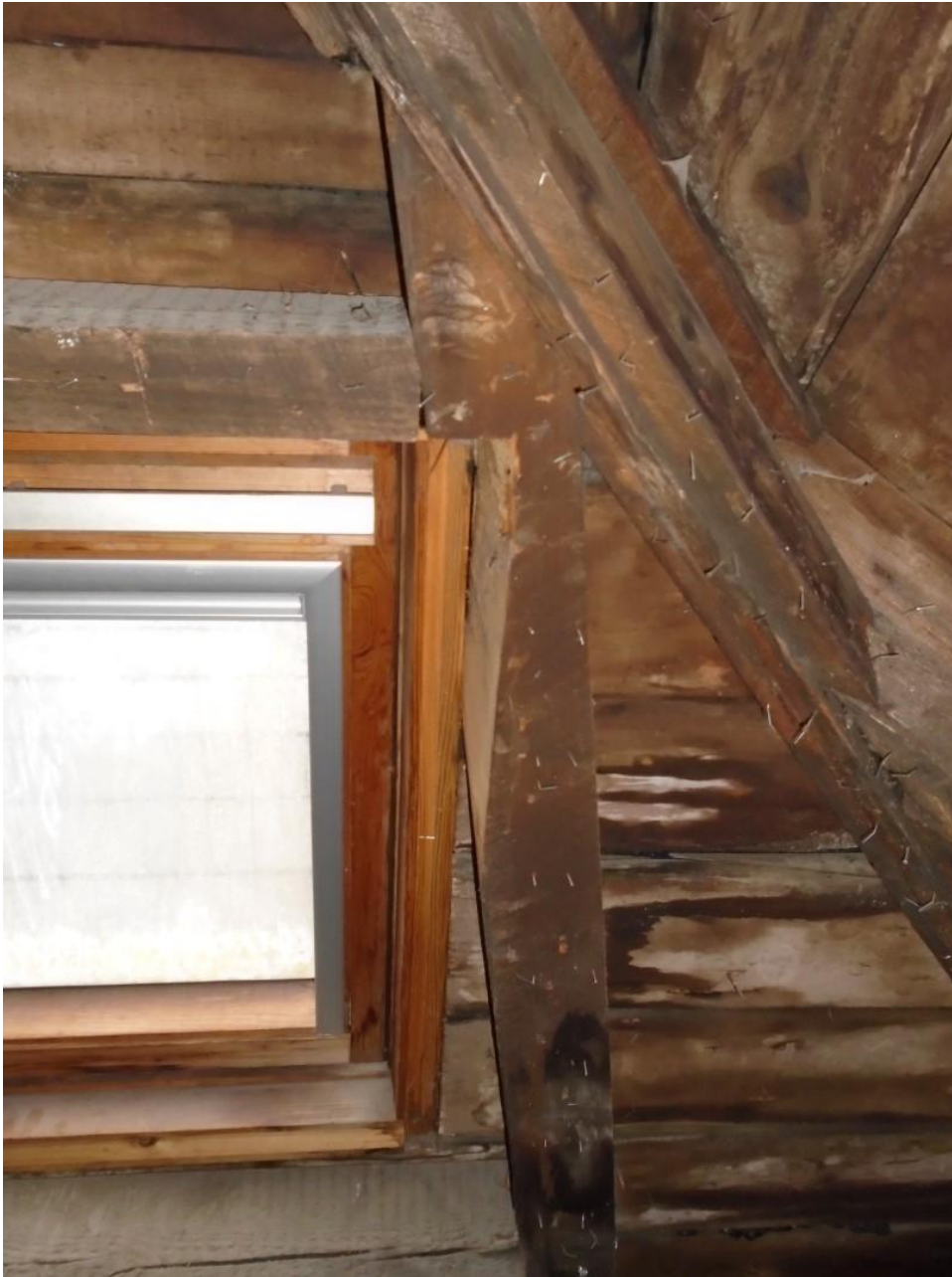
Image 33: Structural integrity of rafter compromised by excessive notching to roof light
