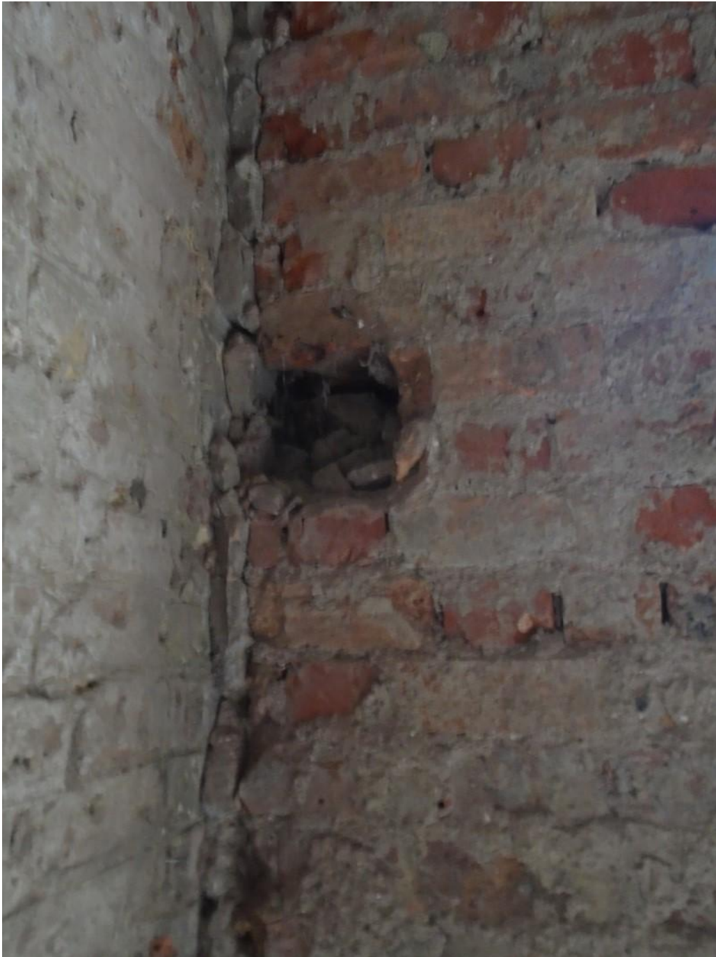
Image 7: Internal view of rear facade inadequately toothed in/tied to party wall – Image 1
