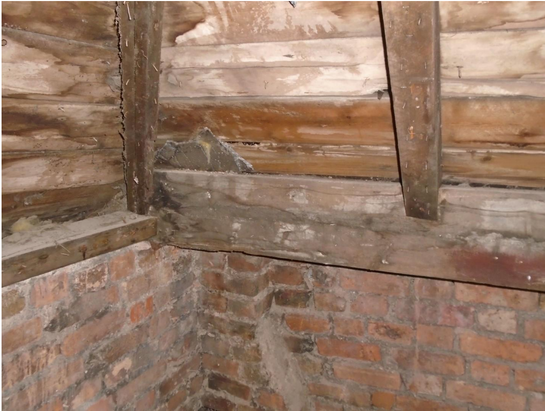
Image 27: Roof waling beam and rafter ends showing signs of rot – Image 1
