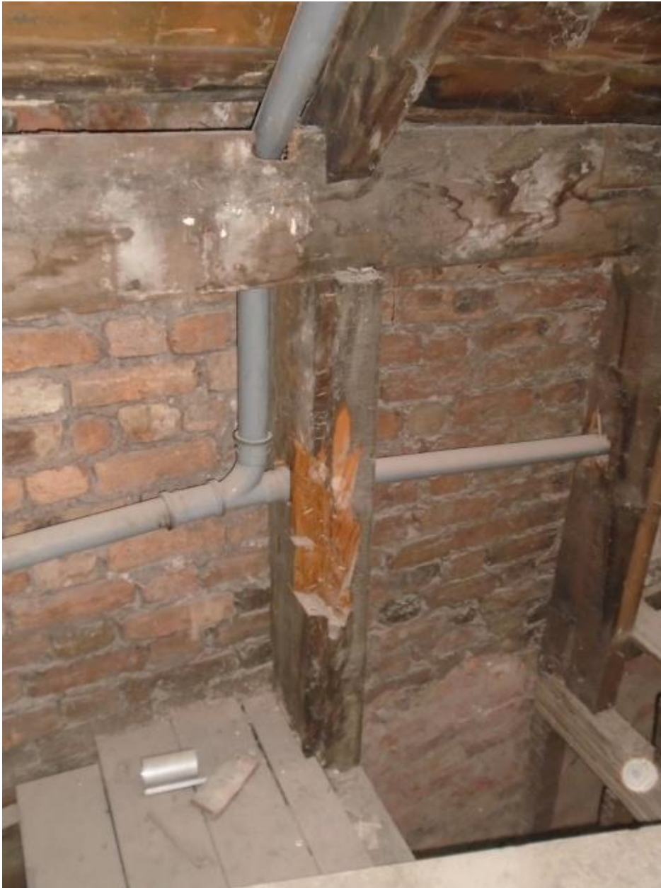
Image 29: Excessive notching to timber prop supporting roof waling beam
