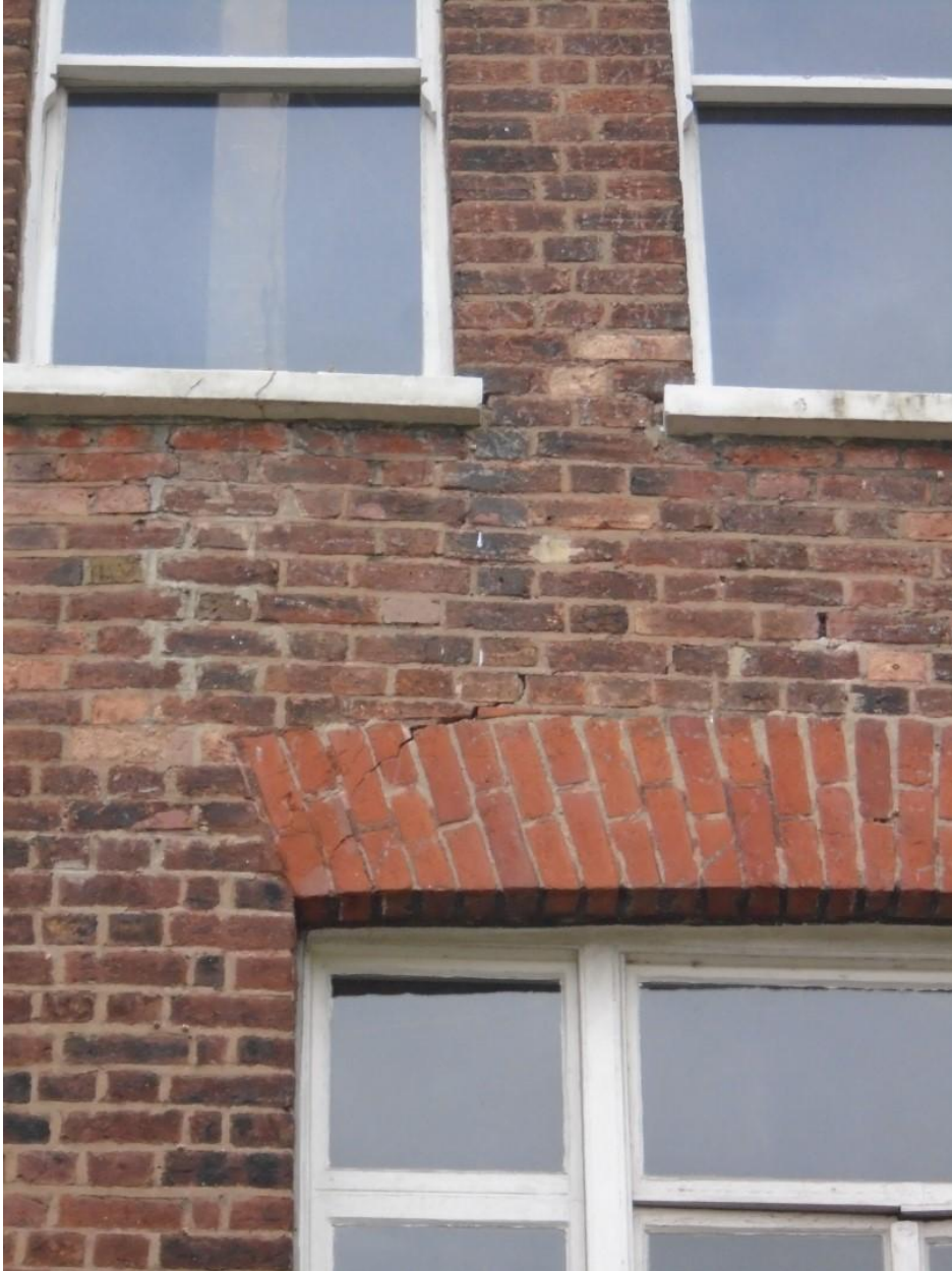
Image 1: Image of cracks in lintel to rear wall due to deformation of the wall/foundation settlement
