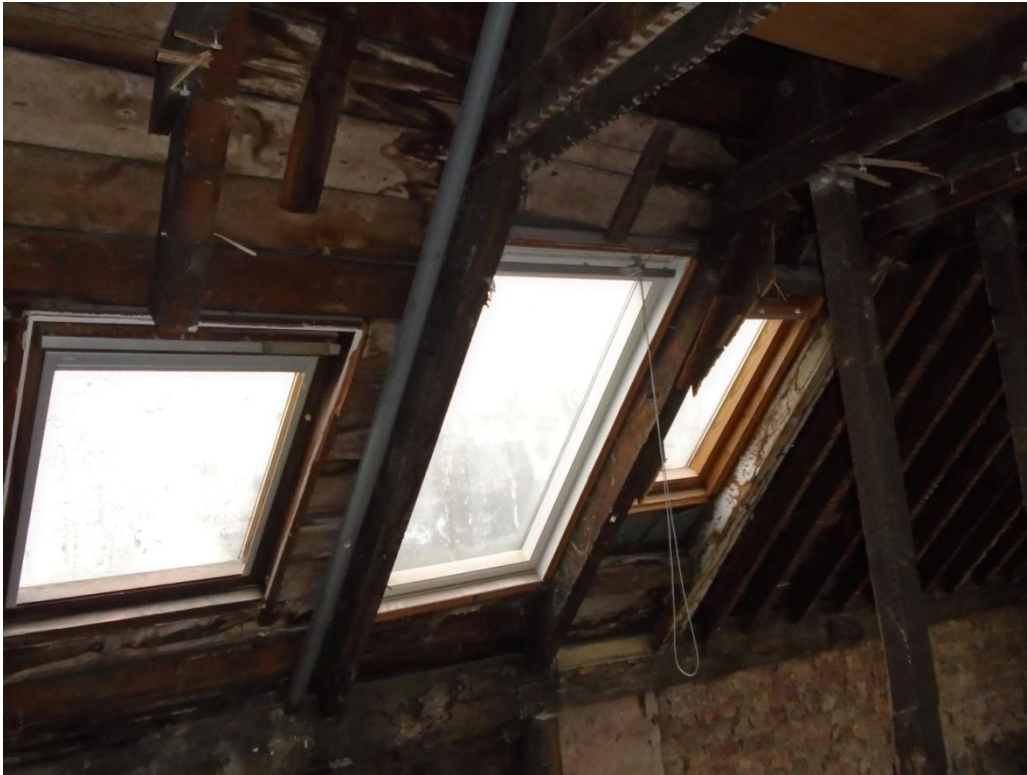
Image 34: Poor condition of roof structure and inadequate trimming around roof lights
