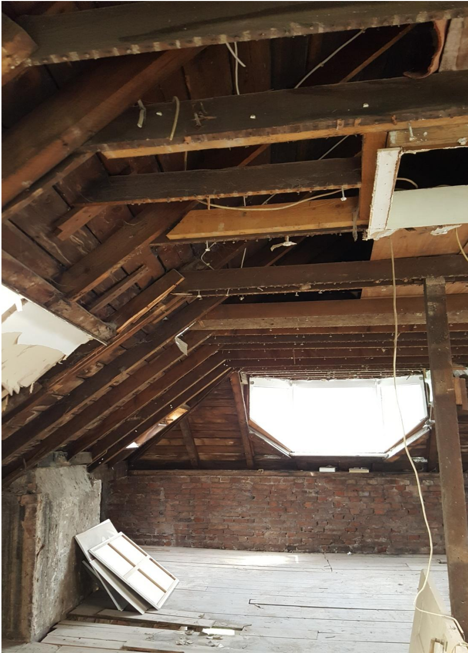
Image 40: General view of poor state of roof construction and sub standard interventions for roof lights
