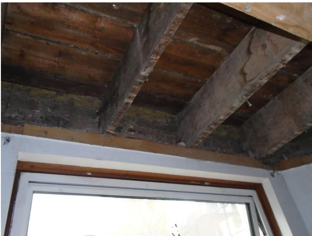
Image 13: Undersized joists and evidence of rot where joists bear on external wall
