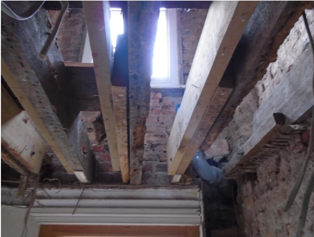
Image 23: Rotten floor joists inadequately spliced – Image 2
