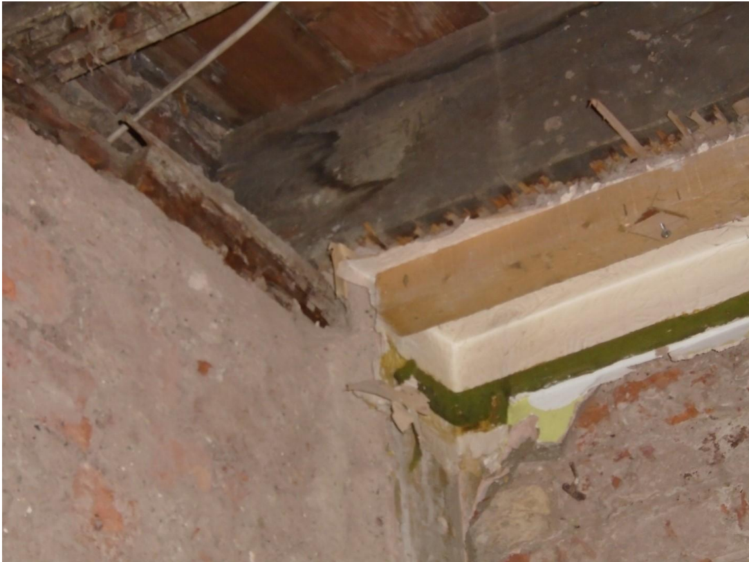
Image 10: Evidence of rot in floor joist ends and timber wall plate
