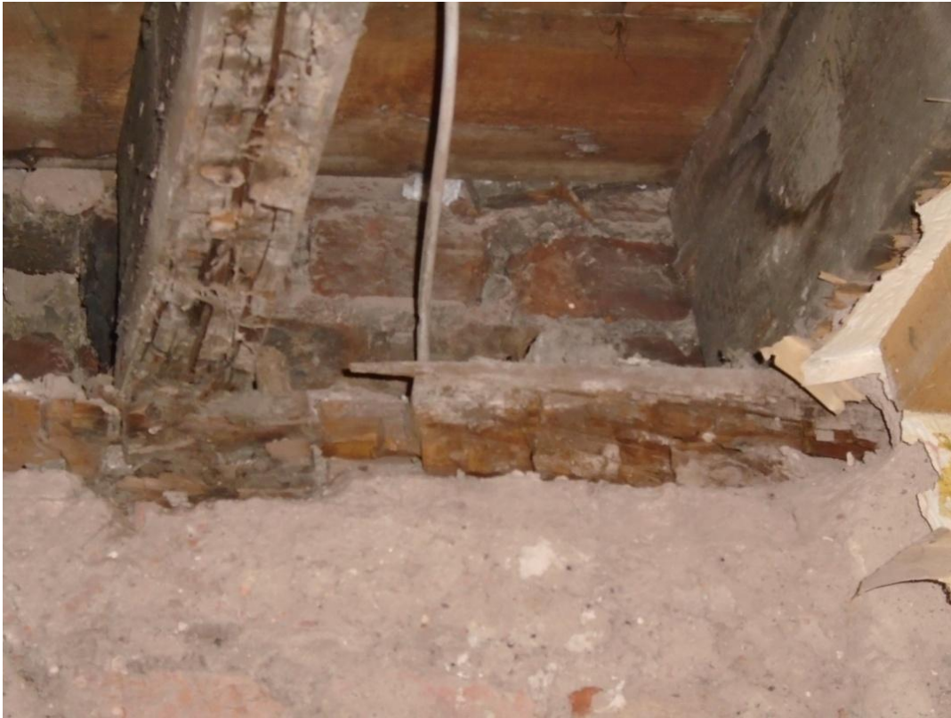
Image 12: Image of rotten floor joist
