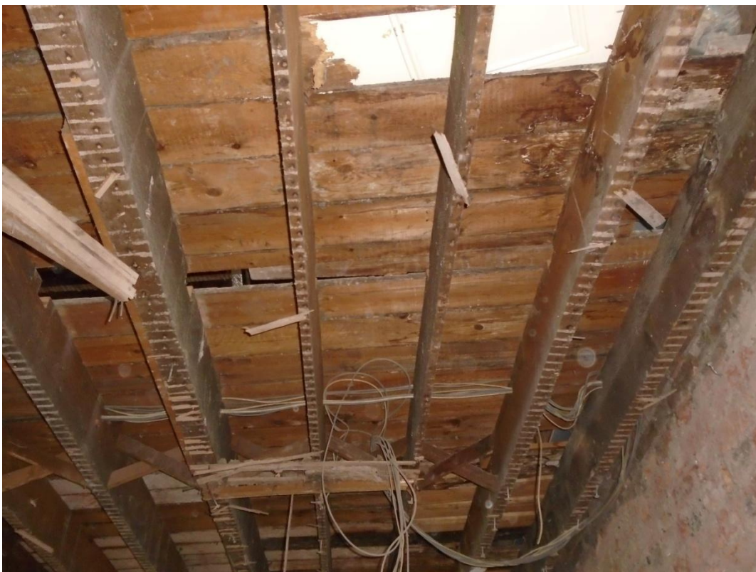
Image 26: Joists inadequately sized
