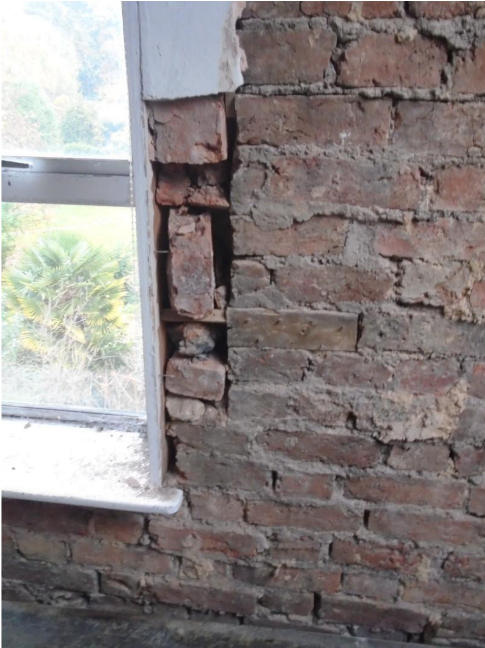
Image 9: Loose brickwork to window reveal in rear facade
