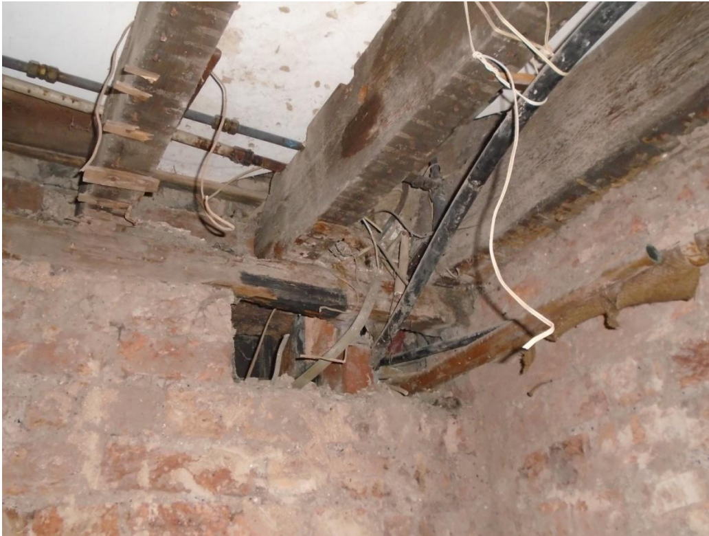
Image 16: Notching of joists and rot evident where joists bear on internal spine wall, general poor condition
