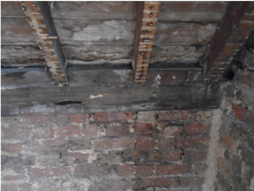
Image 31: Poor condition of brickwork and rot evident in roof waling beam and rafter ends
