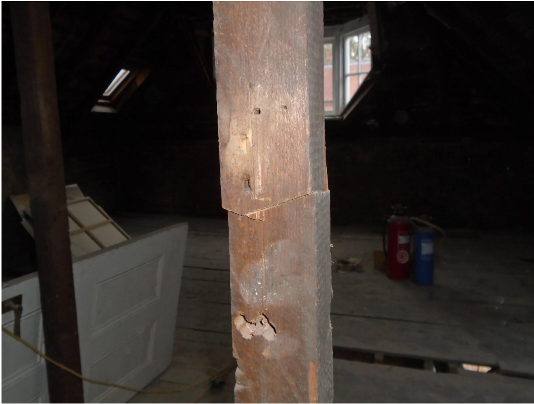
Image 36: Splice in vertical timber prop to roof structure is inadequate and potentially dangerous
