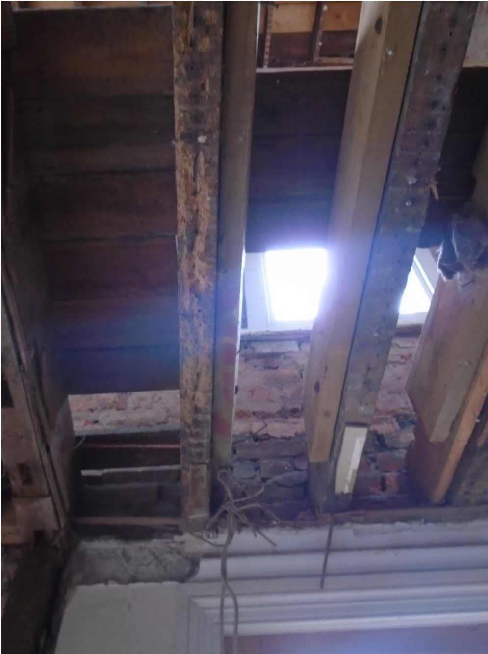
Image 22: Rotten floor joists inadequately spliced – Image 1
