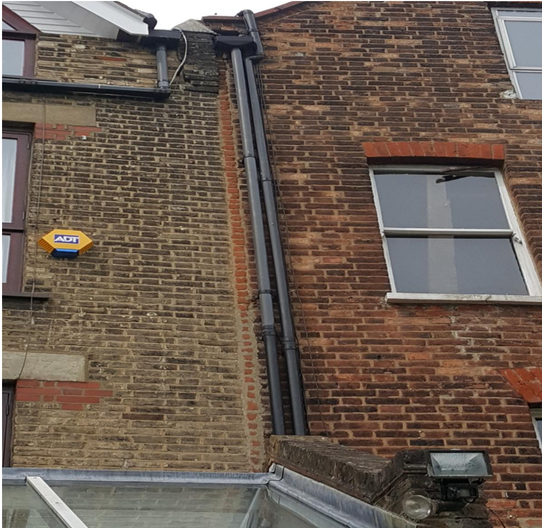
Image 5: Rear elevation showing poor condition of brickwork, sub-standard repairs and different brick bond
