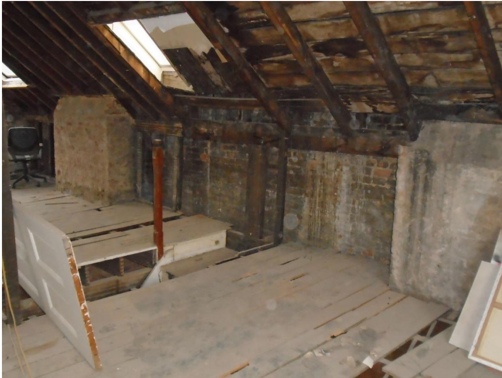
Image 38: General image of poor condition of second floor joists, brickwork, roof waling beam, roof rafters and timber boarding to roof
