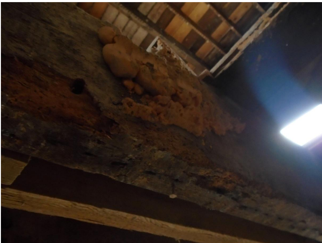
Image 24: Image of rotten joist
