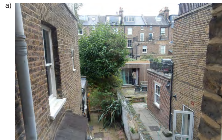
a) Photograph of the existing boundary wall between no. 15 and 17, showing roof terrace at 1st floor to no.17
