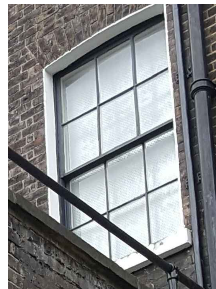
PHOTO 5 No 67 2nd Fl Rear Right Window Window No: WX.2.23
