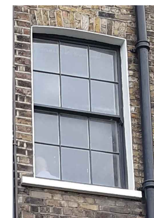
PHOTO 5 No 66 1st to 2nd fl landing window at rear (For GF to 1st FI landing window see Photo 7) Window No: WX.1.04, WX.2.04
