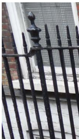
Fig.4a Black iron railings to front lightwell.
