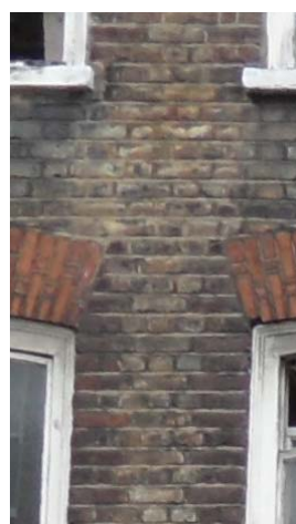
Fig.4b Brickwork on front elevation showing cement
