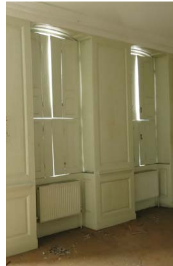
Fig 3m. 39 Great James Street. Existing first floor shutter boxes.
