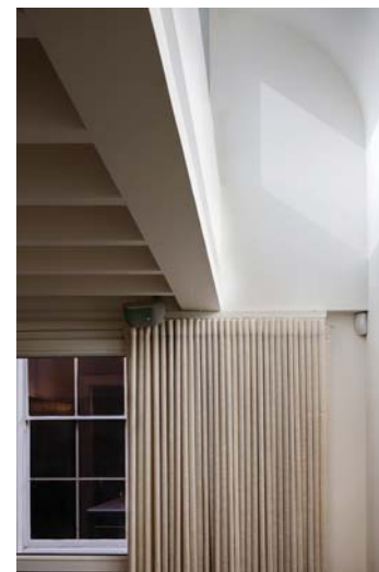
Fig 3aa. Light scoop bringing natural light into lower floors. Prewett Bizley Architects
