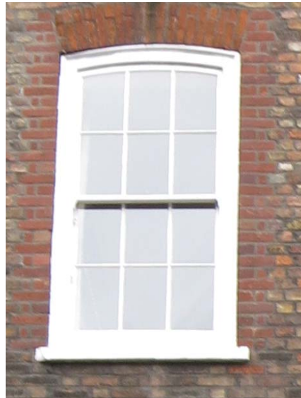
Fig 3vi. Photograph of sash windows with glazing bars at No.38 Great James Street.
