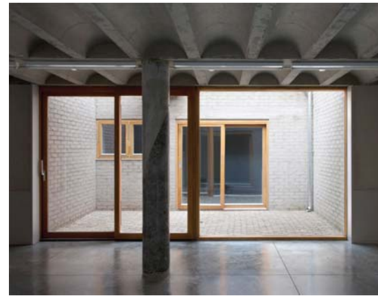
Fig 3viii. Example of timber framed sliding doors. Left: Copper lane, Henley Halebrown Rorrison
