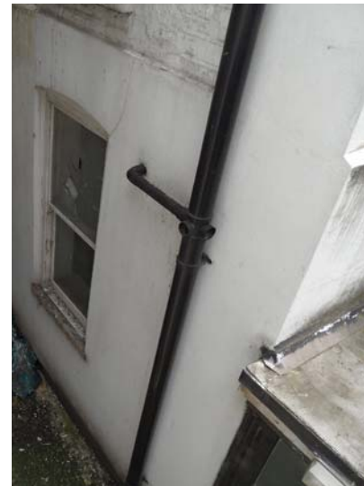
Fig 3iii. Photograph of white painted cement render at rear of property.
