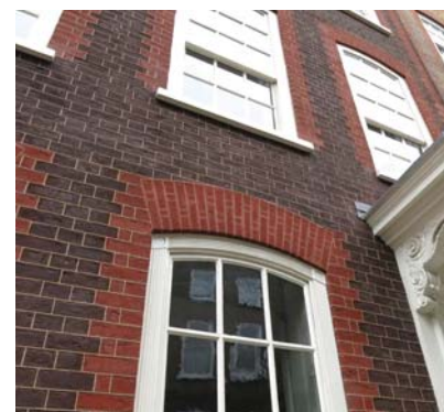
Fig 3a. Example of restored tuck pointing and sash windows with authentic window bars at no.31 Great James Street.
