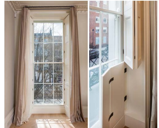
Fig 3n. 16 John Street. Restored windows and shutter boxes. Courtesy of Prewett Bizley Architects.
