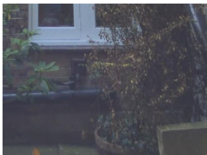
Photo 7: Current extractor outlet between window and drainpipe.
