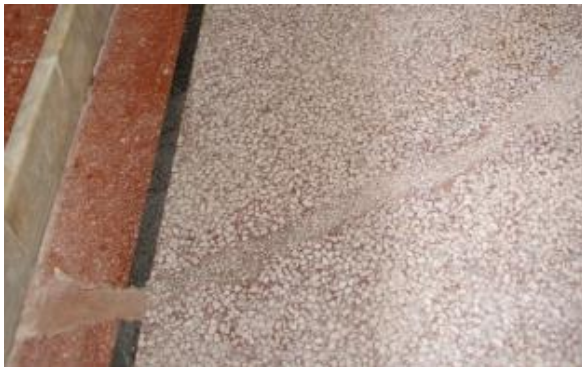
Photo 1: Part of filled crack in living room terrazzo floor
