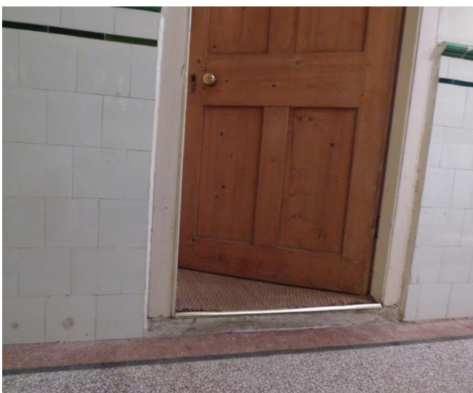
Photo 4: Small 4cm step from terrazzo floor in current kitchen up to concrete hall floor - the cause of many trips
