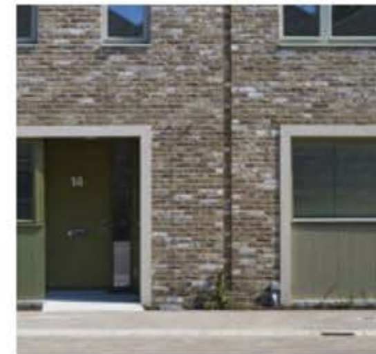
Precedent: AHMM - Anne Mews. Reconstituted stone used to subtly pick out entrances
