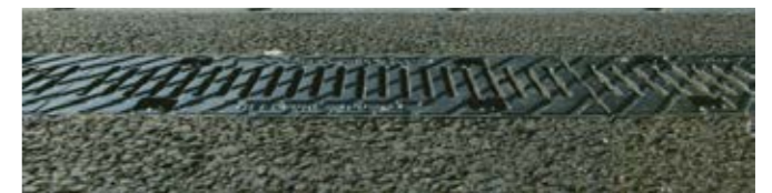
C1 & C2 - Drainage channels
