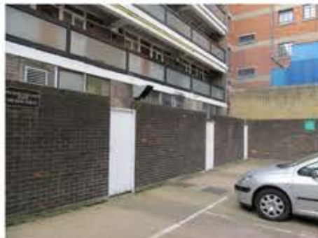
4- There is currently no overlooking of the existing parking area at ground floor level. The wall is dominated by rear access arrangements to the retail units at ground floor.
