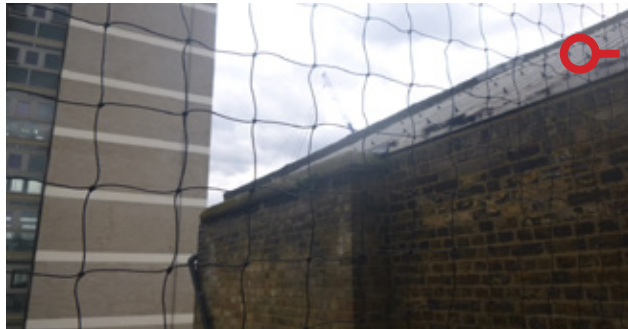
The roof contains asbestos and must be replaced.
