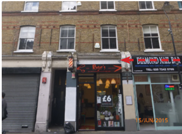
The shopfronts are in a poor state of disrepair. The proposal includes for an indication of the potential upgraded shopfronts (please see section 5.12)
