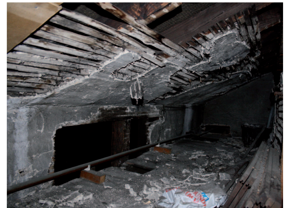
Existing condition of roof structure and fabric viewed inside the eaves storage showing degraded lathe and plaster linings..
