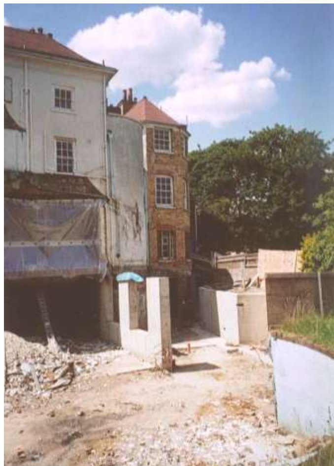
Fig.29: A view of the 2003 excavation works and new construction on the southeastern side of the house
