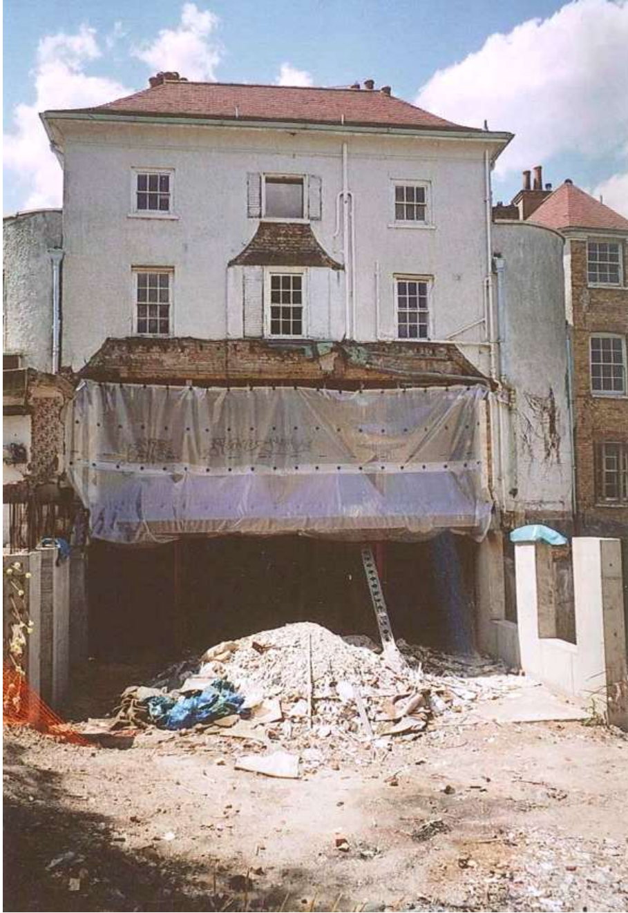
Fig.27: A more detailed view of the 2003 excavation works in progress on the eastern side of the property
