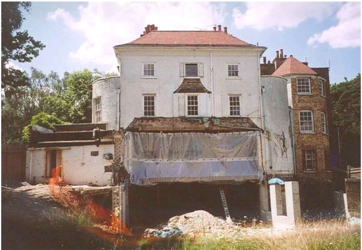
Fig.26: A similar view taken in 2003 during the preliminary excavations for the new lower ground floor
