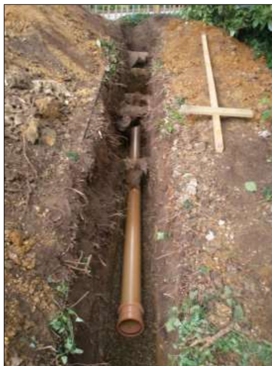
Services image 2: Continuous trenches dug by hand so that important roots can be retained (with the service ducting threaded beneath) is an effective means of minimising damage (note the ground protection boards with soil piled on top on the left).
