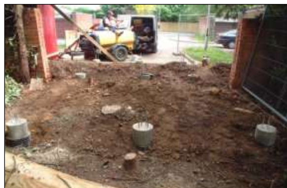
New structure image 8: Piles can also be used to support bridges across sensitive RPAs, but the temporary ground protection has to be removed before the main structure is either imported in or cast on site.
