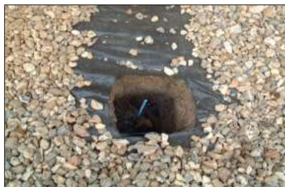
New structure image 6: Ground protection must be used to spread the load of the piling rig once excavation has confirmed that no substantial roots are in the preferred pile location.
