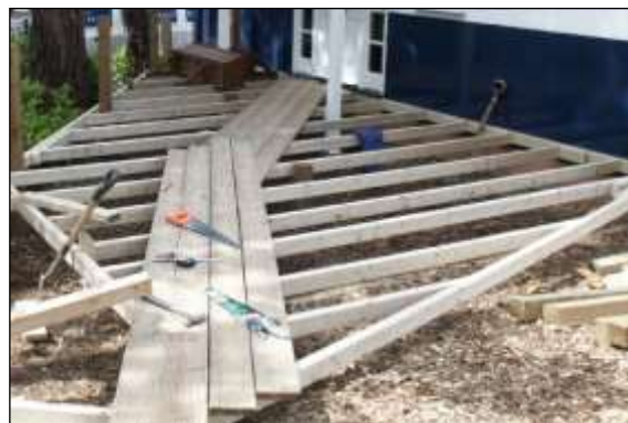
New structure image 2: This deck supported above the ground on small posts provides a low-impact alternative to conventional stone patio surfacing in RPAs.
