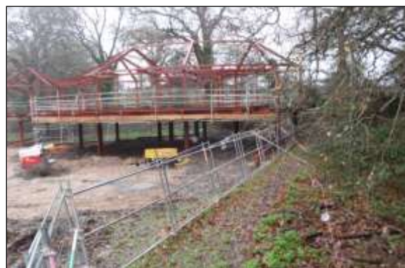
New structure image 4: It is possible to support very large structures on piles within sensitive RPAs without any significant adverse impact on tree roots.
