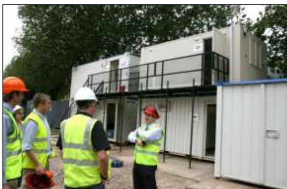
Ground protection image 7: A combination of retaining existing surfacing and using temporary construction cabin accommodation can be a very effective means of preventing damage to sensitive areas.
