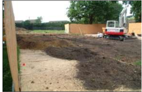
Ground protection image 2: Spreading soil excavated from footings is an effective way of buffering the plywood surface from the wear of light vehicles.
