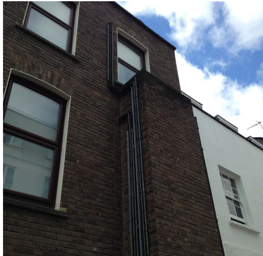
Surface mounted condensate pipework clutter - Rear
