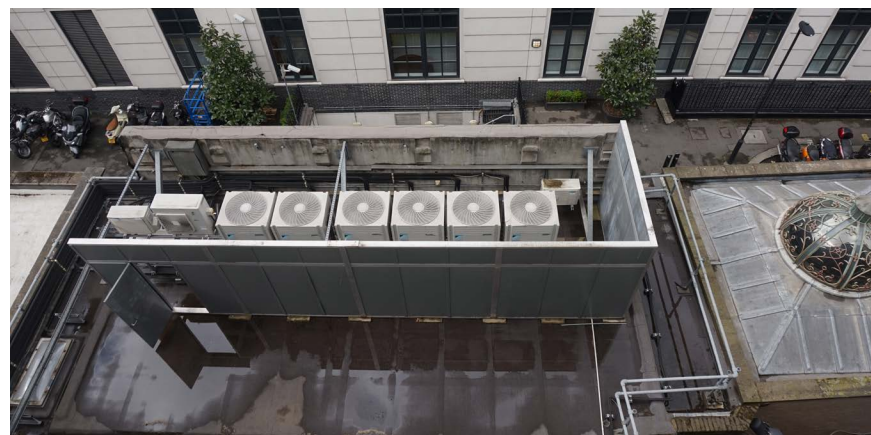
2F Plant Enclosure and terrace
