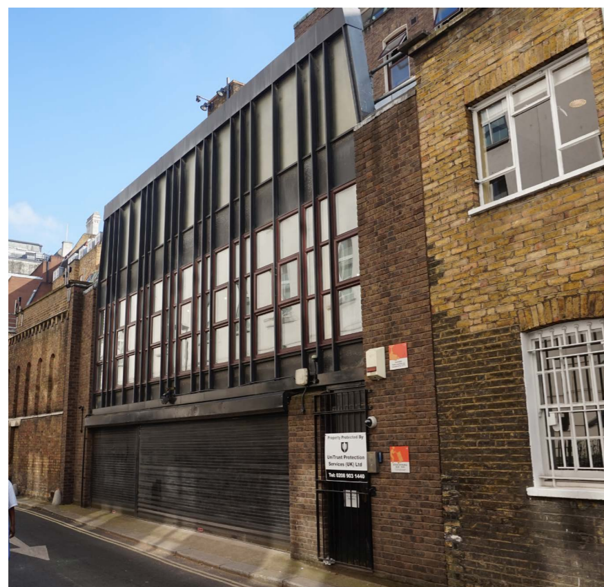
Metal shutters to garage door and guarding
