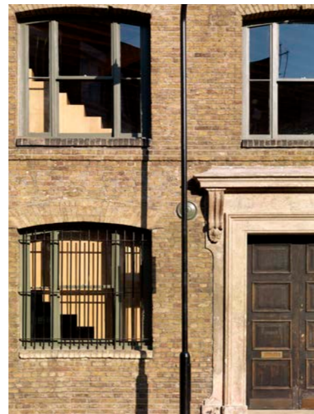
Fig. 34 - Period warehouse refurbishment. Brick cleaned of all paint and lightly sootwashed (B). Original timber windows reinstated and painted (C).
