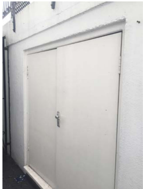
Water Tank Store
