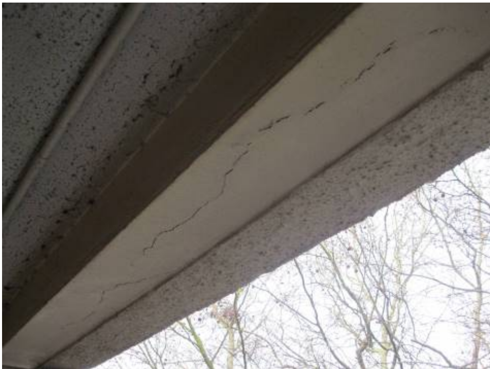
Photograph 24 Cracking to access balcony ring beam soffit
