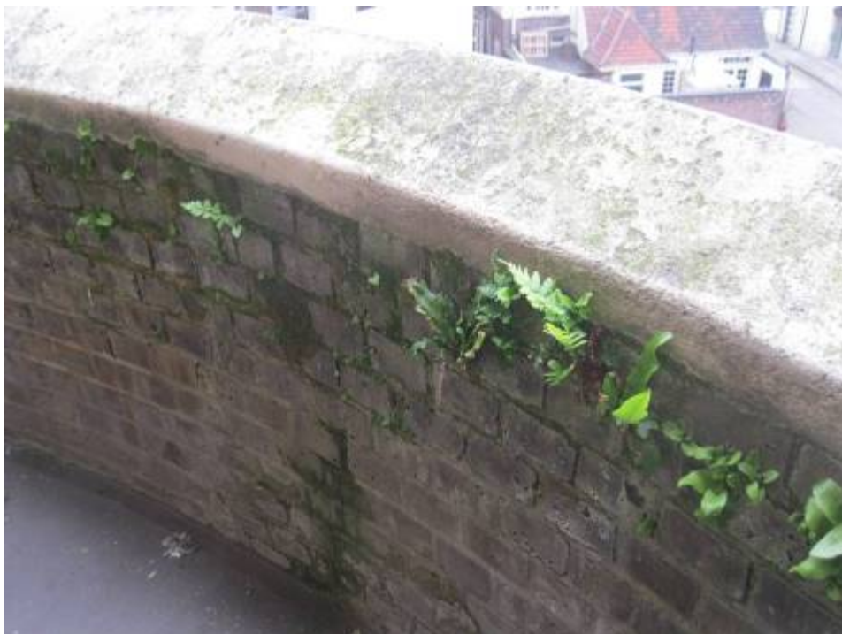
Photograph 36 Poor condition of access balcony parapet
