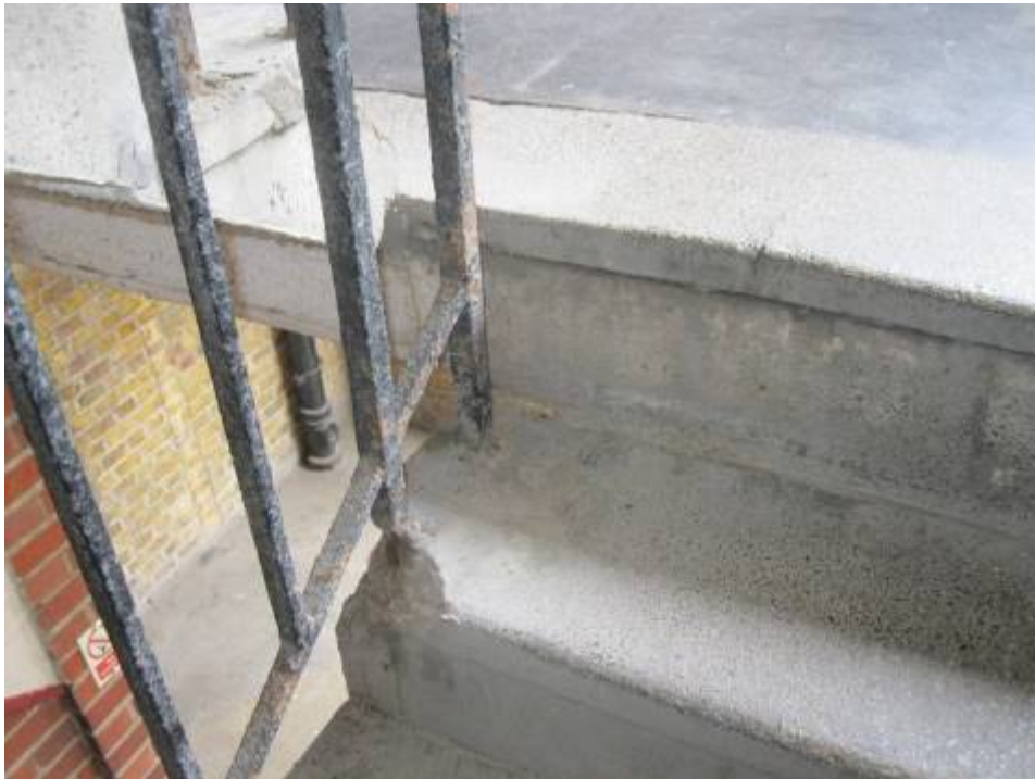
Photograph 35 Communal stair repairs and redecorations required
