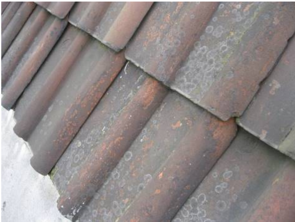
Photograph 12 Existing tile condition
