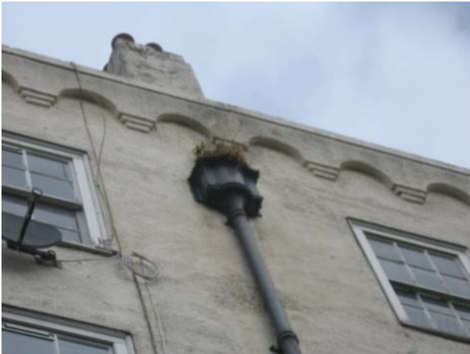
Photograph 33 Blocked rainwater hopper
