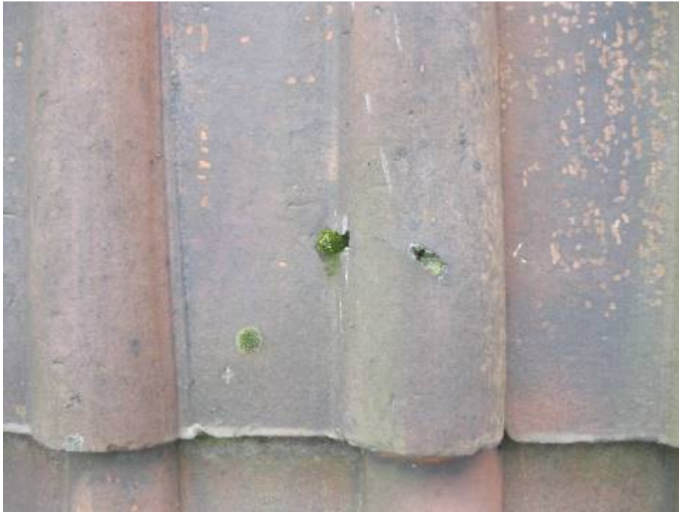
Photograph 13 Existing tile condition
