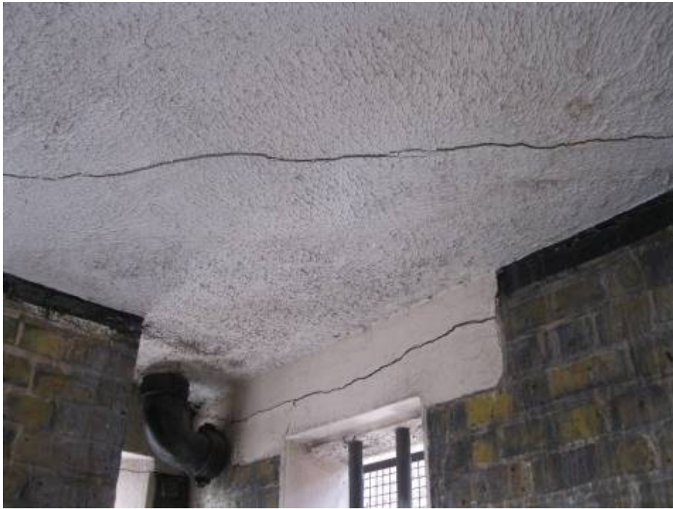
Photograph 37 Structural movement in 135 – 180
