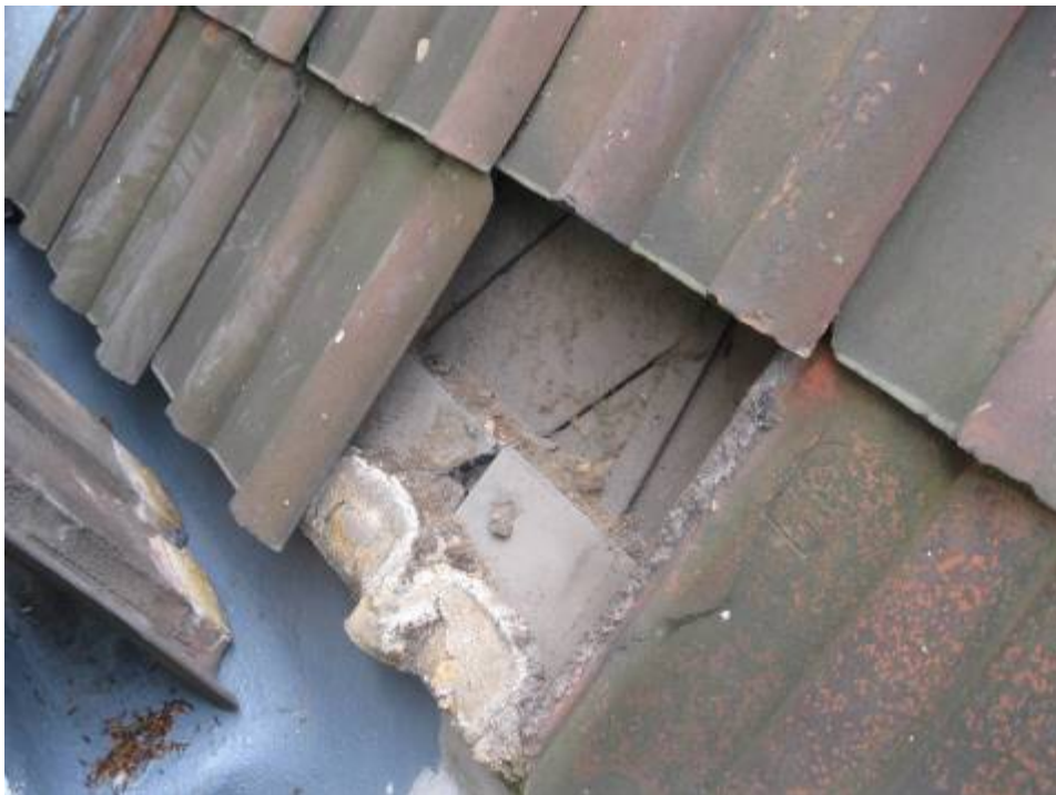
Photograph 10 Tile removed, no sarking felt
