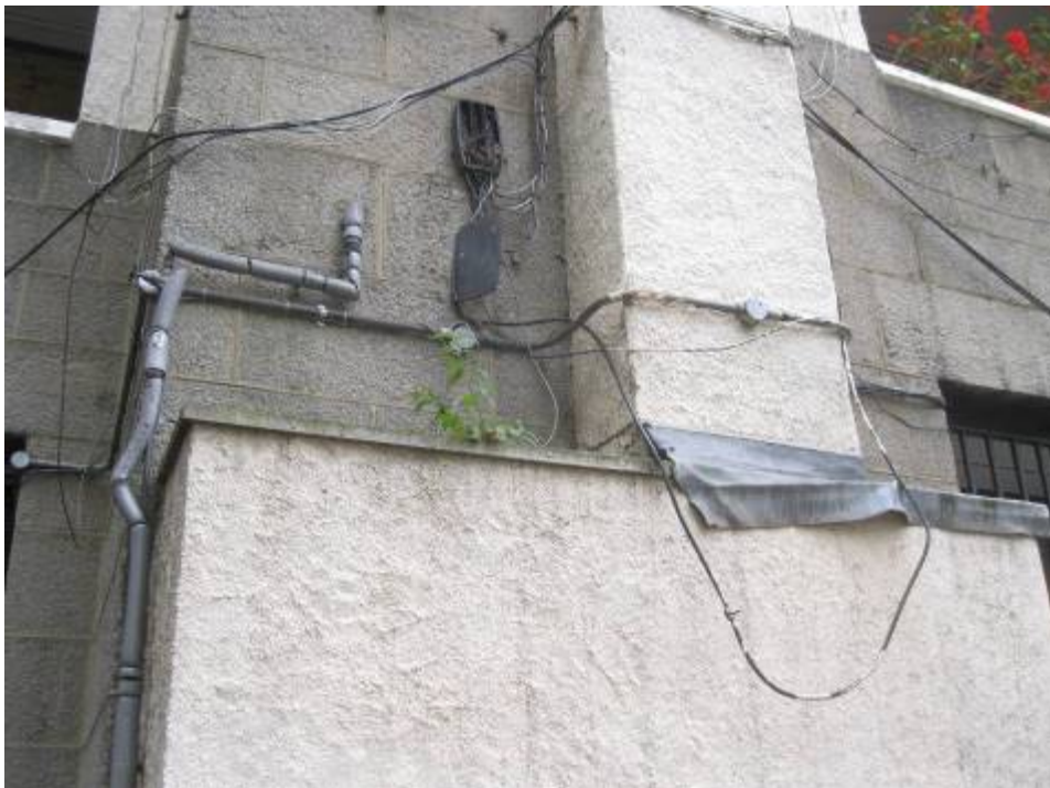
Photograph 38 Damaged flat roof, cable condition, and poorly insulated water supply
