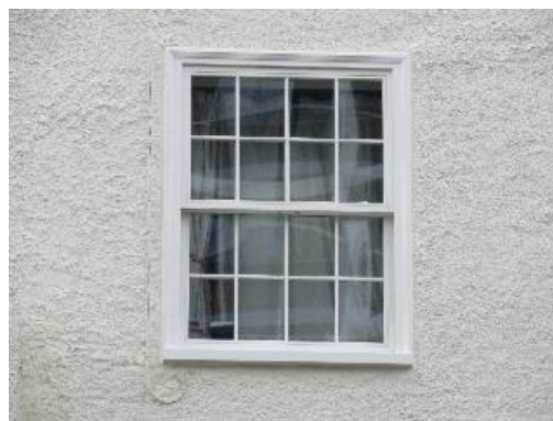
Proposed replacement sash window type as fitted in adjacent Levita House block
