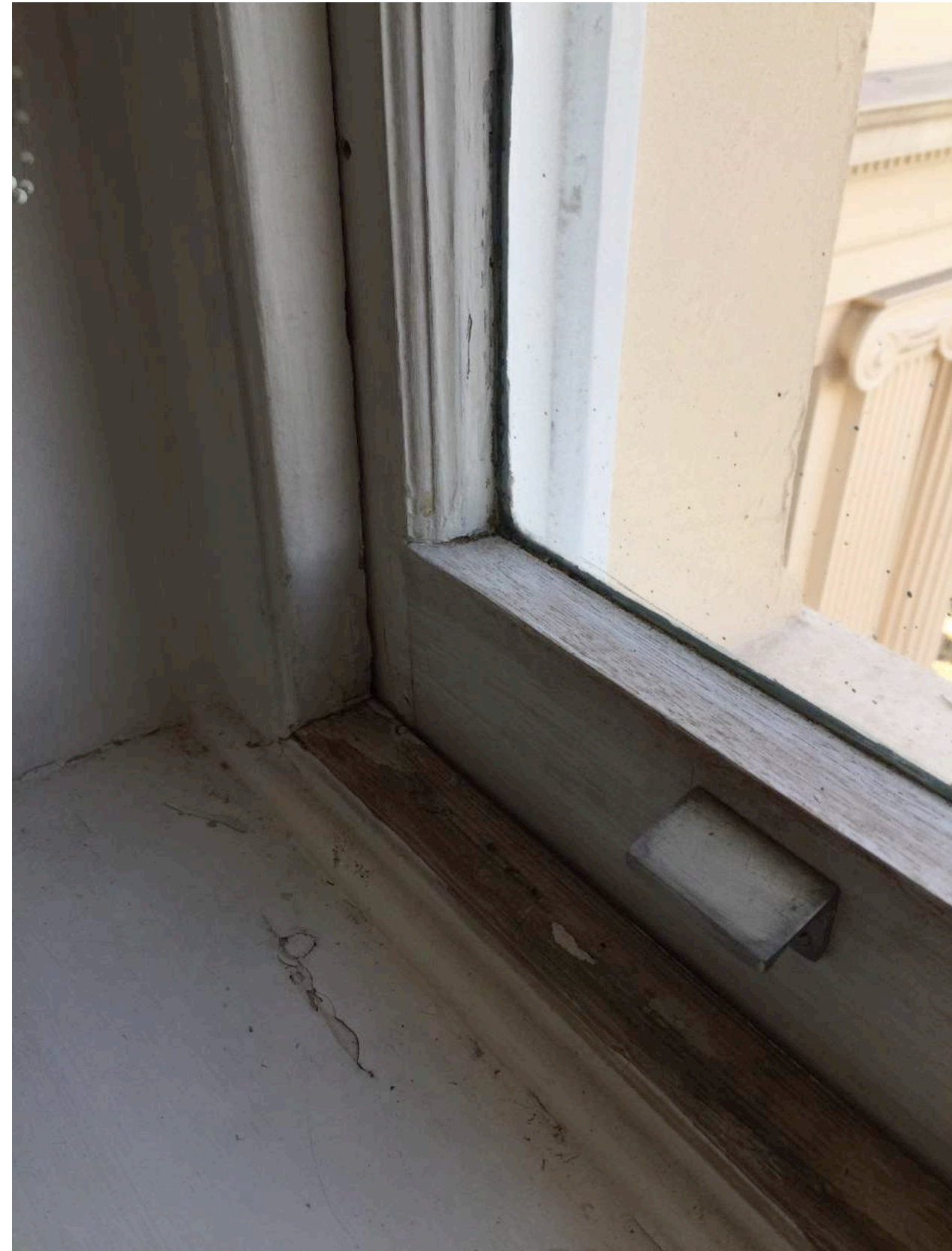
SASH WINDOW REPAIR incorrect bottom rail detail to be rectified
