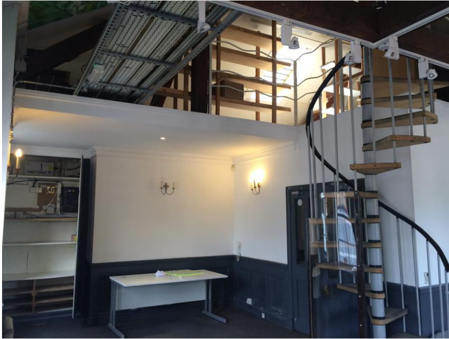
Figure 9: Tack Room: first floor: north bay. The partitions and mezzanine floor are modern and to be removed.
