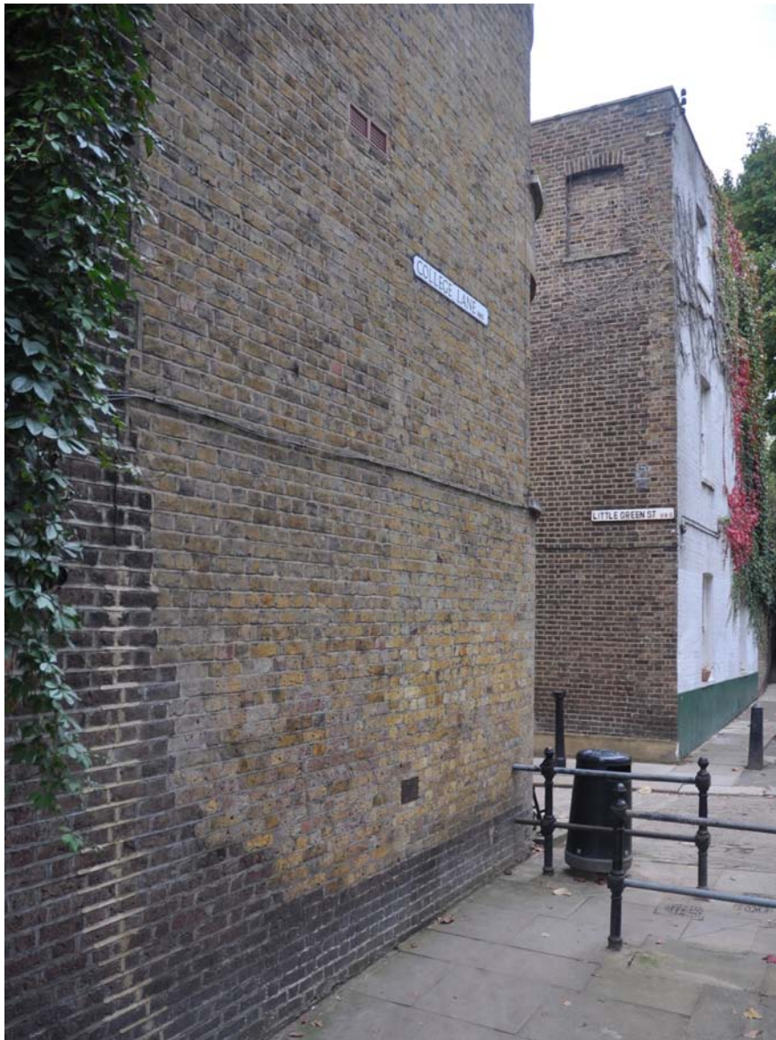
Figure 17/ Front and side elevation of No. 8 and side elevation of No. 9 showing possible WWII bomb damage, 2016.
