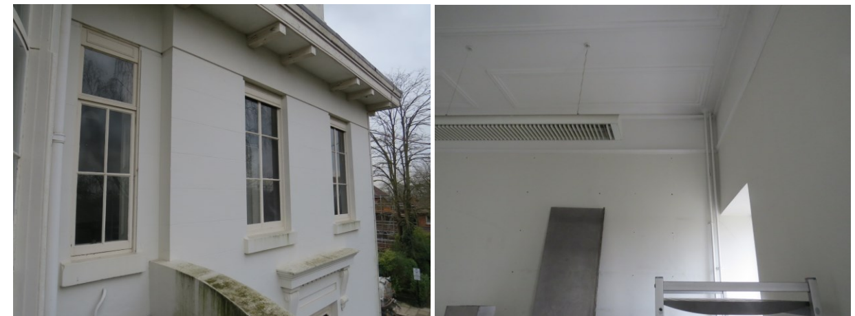
Figure 62. (Left) A photograph of the west elevation taken from a location on the balcony to the bay window. The central window is divided internally by the later partition. (Right) The internal partition which cuts the window internally.
