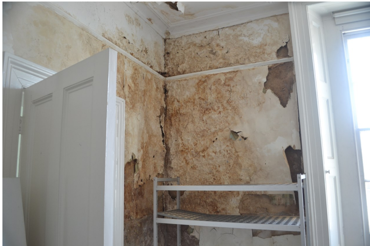
Figure 68. An image of the damage caused by water ingress at the first floor level.
