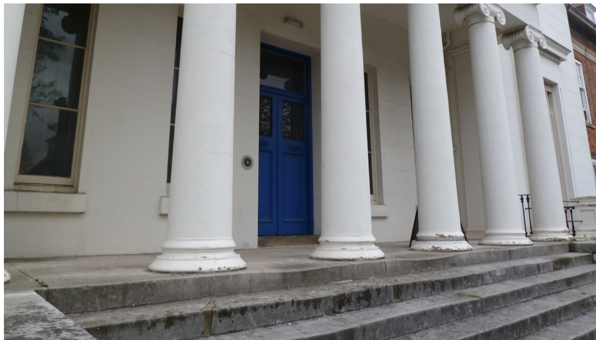
Figure 54 The entrance steps to Kidderpore Hall accessed from Kidderpore Avenue. The plaster render and the stonework of the steps are in need of refurbishment.
