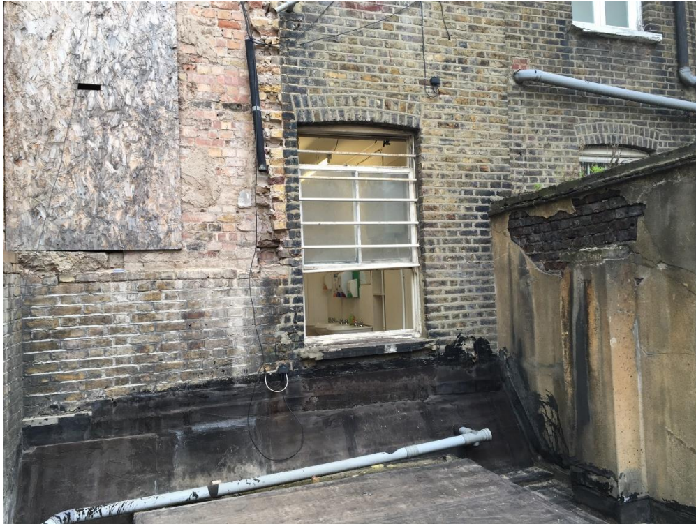
Photo 3: View of the rear of Nos.60-61 TCR at first floor level in a poor state of repair
