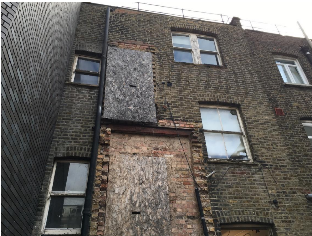
Photo 4: View of the rear of the upper floors at No.61 TCR in a poor state of repair
