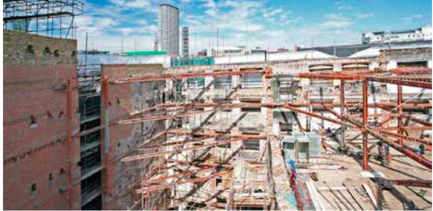
14. Photograph showing the damage to the Seven Dials Warehouse, c.2000 (AKT II)
