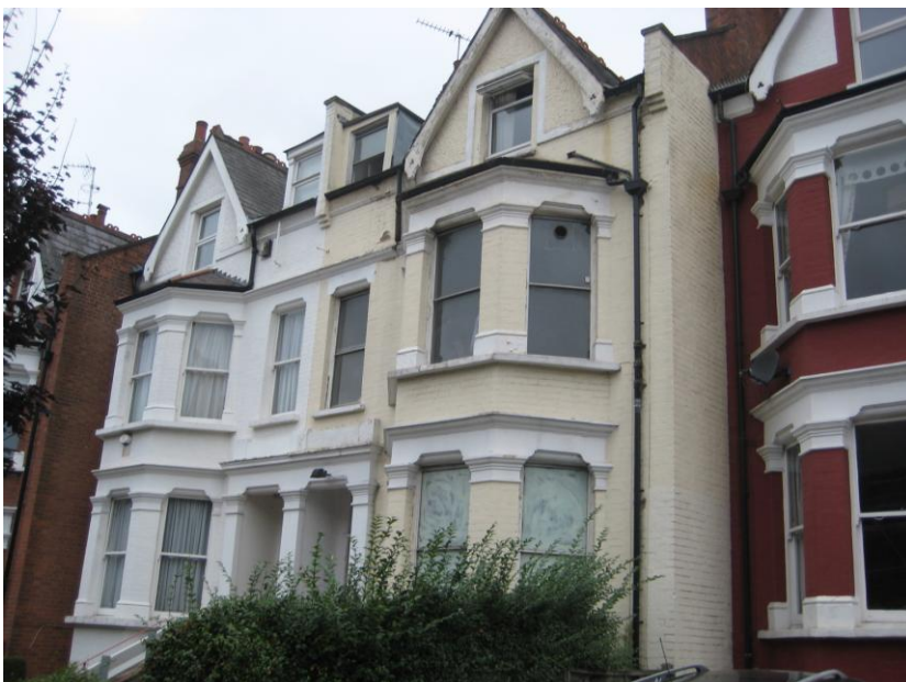
Front view of the property, showing the existing change in window character between 7 Lyncroft Gardens and the properties on either side
