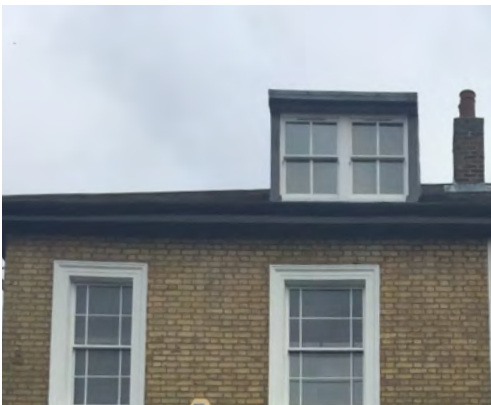
Image 1.04- 20 Rochester Square- Existing front double lead clad dormer
