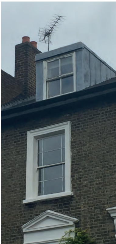
Image 1.01 - Existing front elevation of the house with a single lead clad dormer
