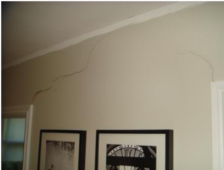
FIGURE 04 Crack damage to the garden flat front left bedroom.
