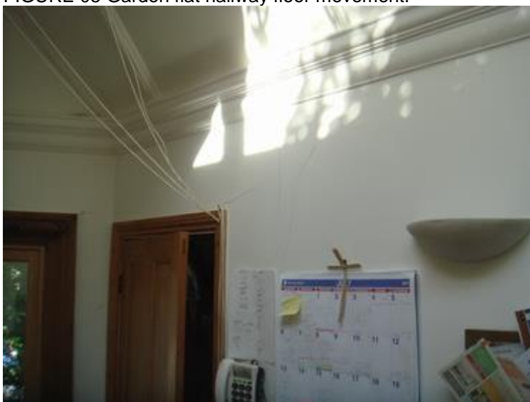
FIGURE 06 Ground floor flat crack damage recorded to the front right kitchen.
