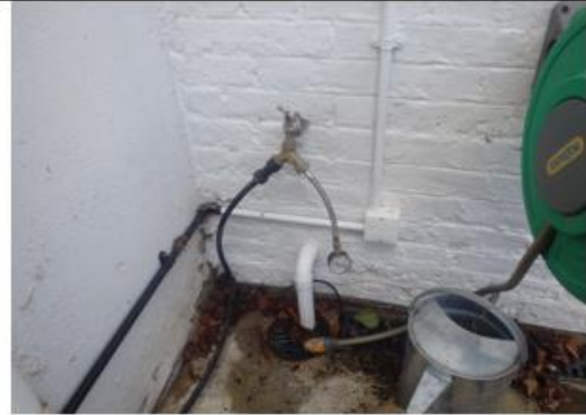
3. FWG1/Mains water pressure test.
