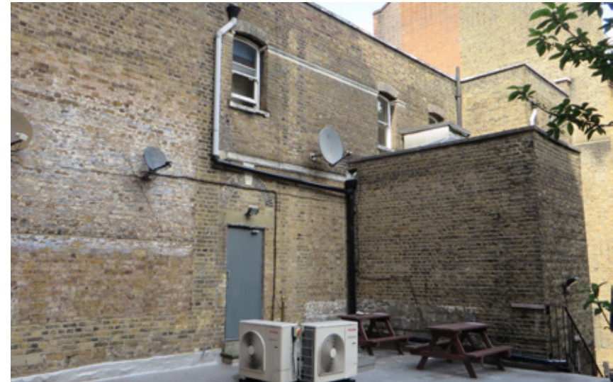
View looking north-east at first floor level to the rear of 125 Clerkenwell Road. Note lack of features, poor quality of brickwork, haphazard rear extensions and drainage runs.
