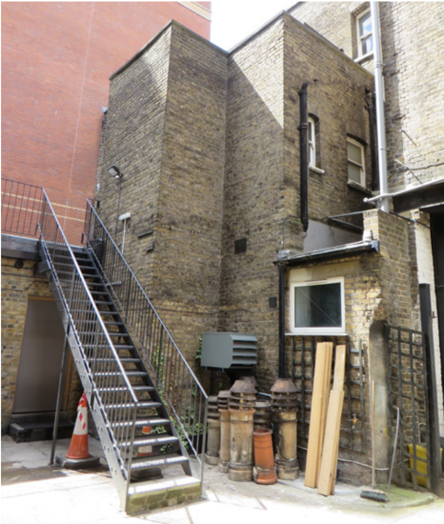
View looking north east from ground floor rear court yard. Note unattractive haphazard rear extensions, poor quality of brickwork and absence of architectural features of any merit.
