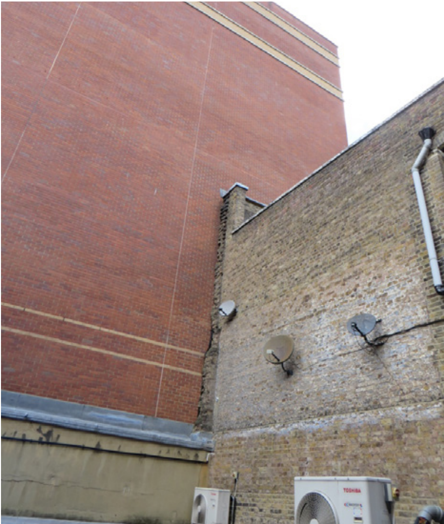
View lookinh north east from first floor level to junction of rear of 125 Clerkenwell Road and 127 Clerkenwell Road. Note poor quality of brickwork, especially snapped headers at junction of two properties, and absence of architectural features of any merit.
