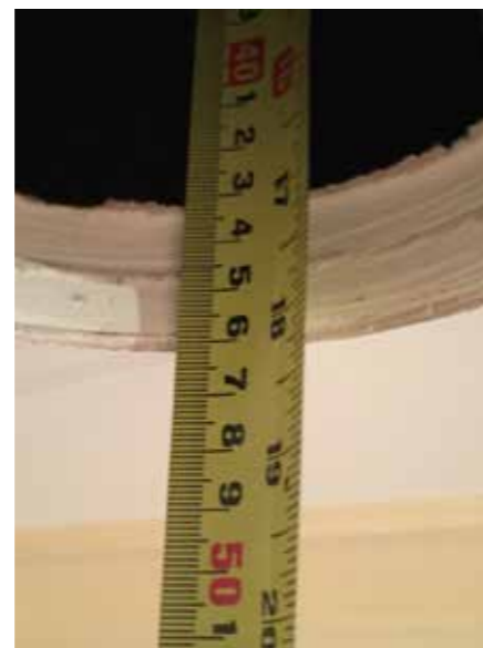
Current Hallway Non Original Double Plasterboard Ceiling.
