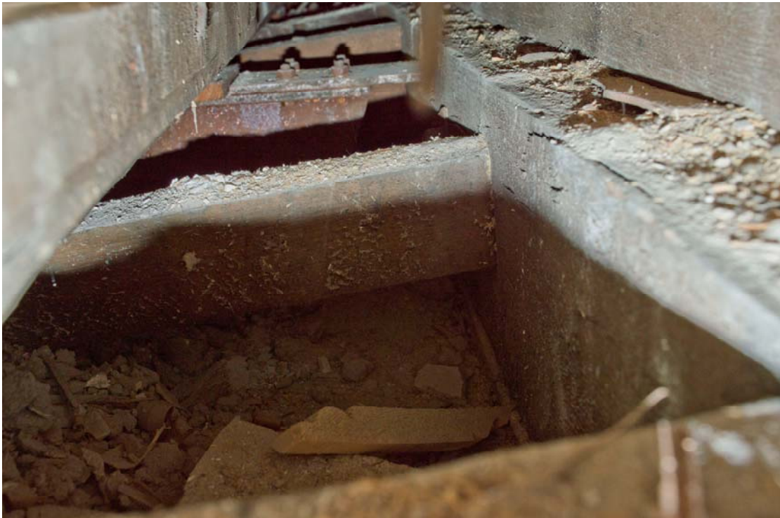
Structure of the second floor (front range), looking north-east along the joists. Note the corroded iron plate running perpendicular to the main timbers.
