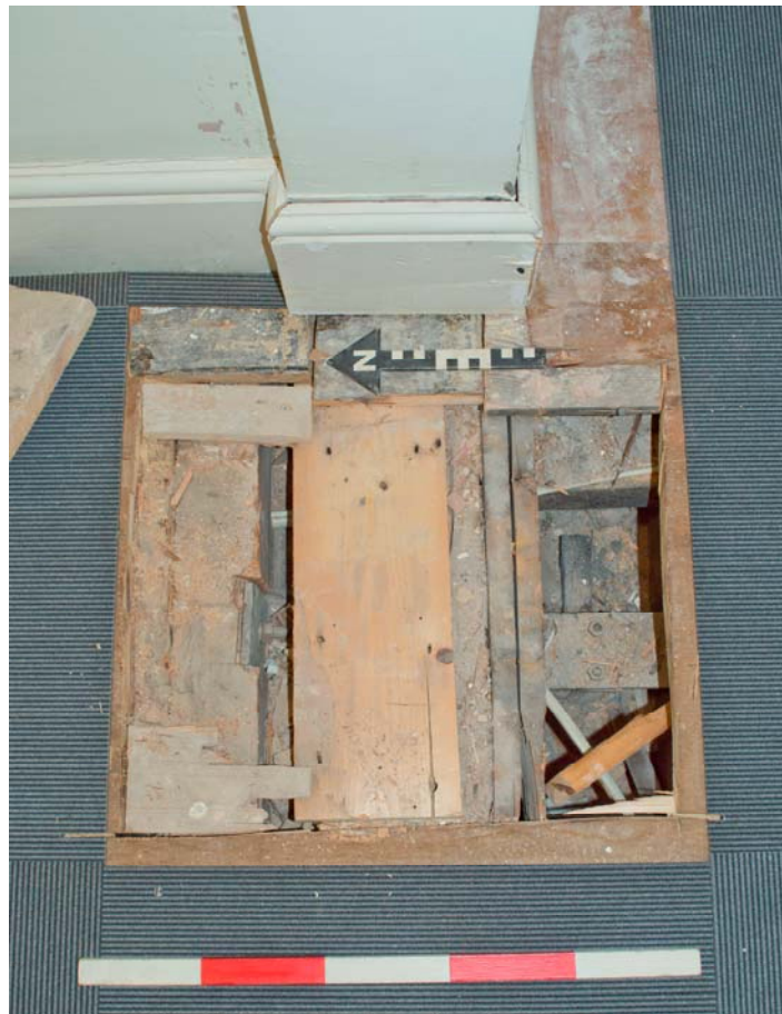
Structure of the second floor (front range), looking north-east. Note the steel plate running perpendicular to the main timbers.
