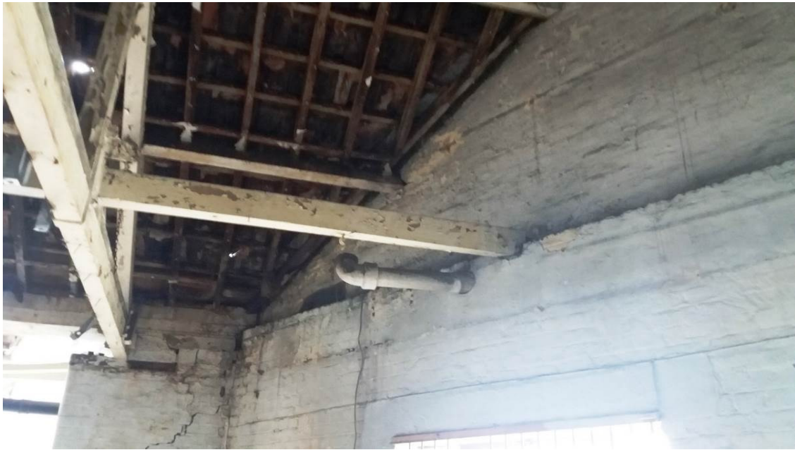
P28 – Inadequate restraint to existing masonry walls
