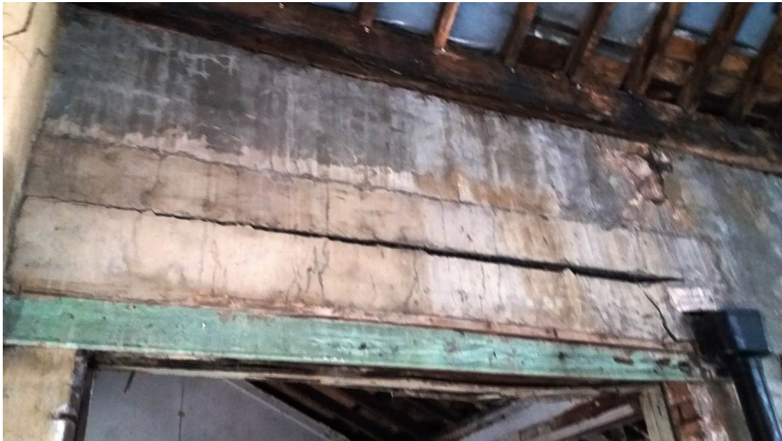
P12 – Wet rot to wall plate and rafters due to waterproofing failure
