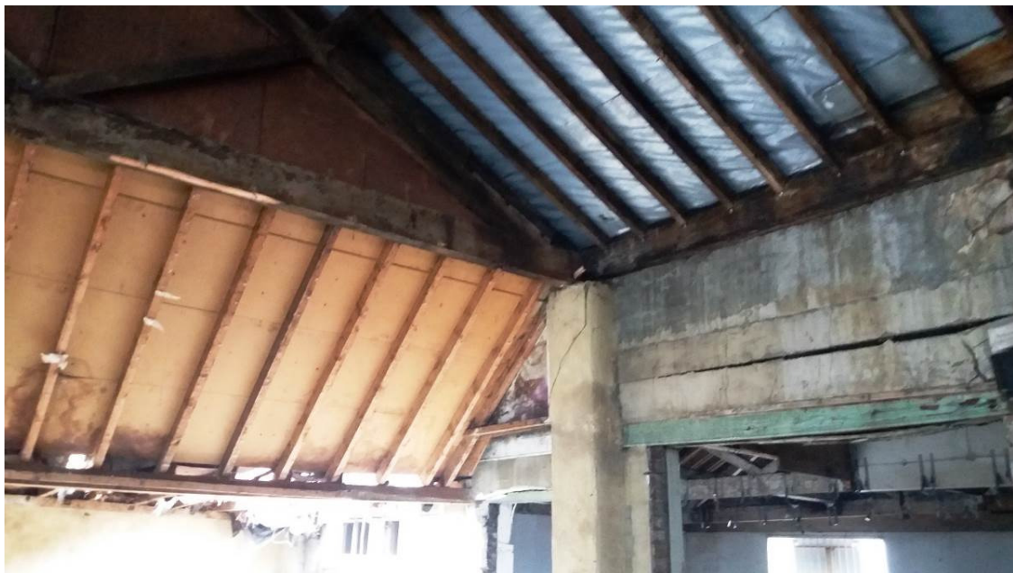
P09 – Water ingress to existing roof
