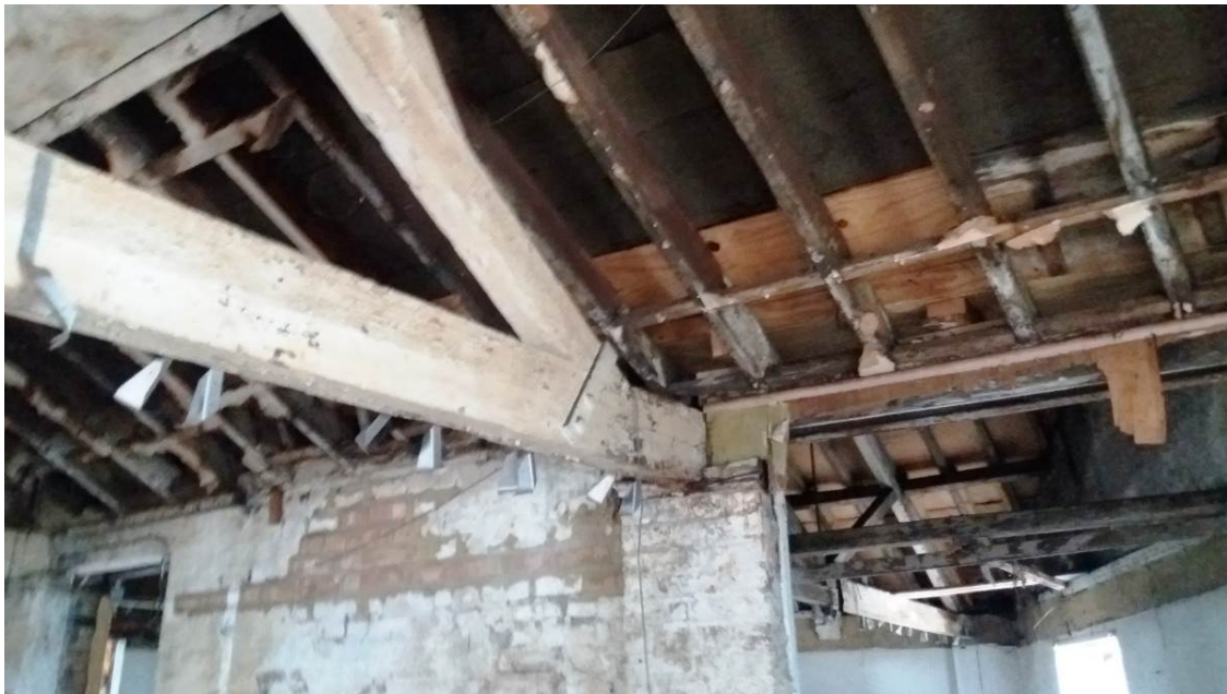
P19 – Inadequate bearing of roof truss
