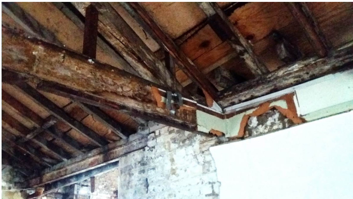
Photo 17 – Rotting roof boards, rafters, wall plate and trusses due to water ingress
