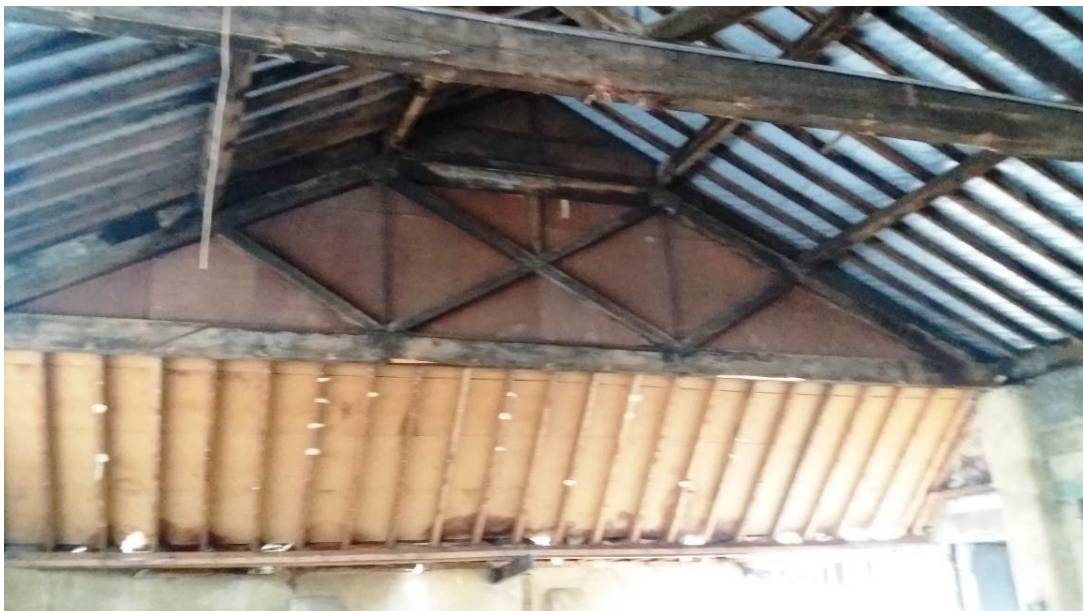
P31 – Internal view of garage roof. No roof bracing present.
