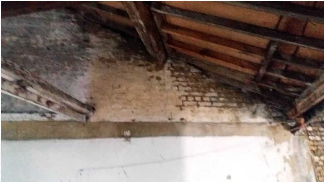
P21 – Water ingress due to failed waterproofing detail impacting masonry walls
