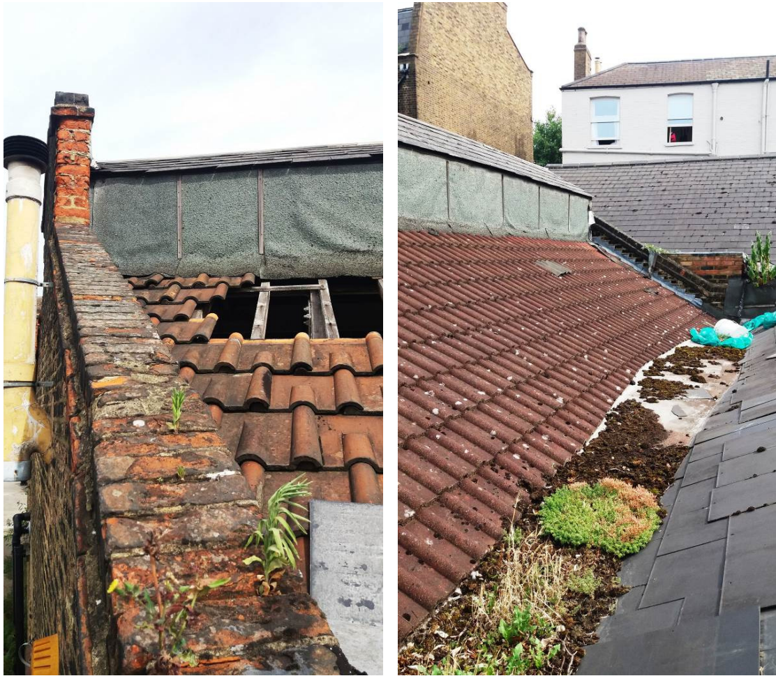
P03 & P04 – View from roof level showing damage and dilapidation of roof
