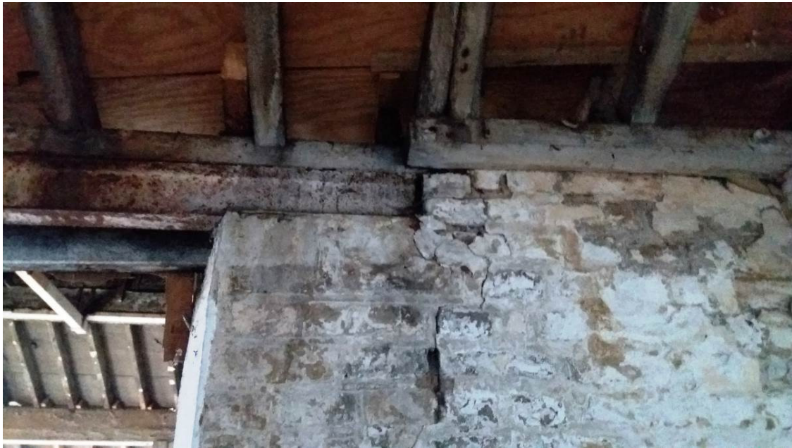
P18 – Cracking of masonry below caused by inappropriate bearing of roof member. Corrosion of existing steel beam
