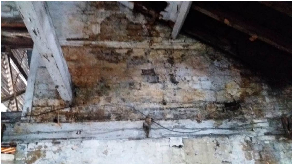
P13 – Deterioration of fabric of structural walls due to roof failure
