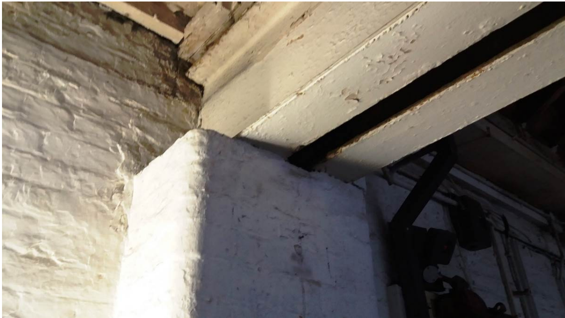
P24 – Corrosion and flaking paintwork to supporting steel beam
