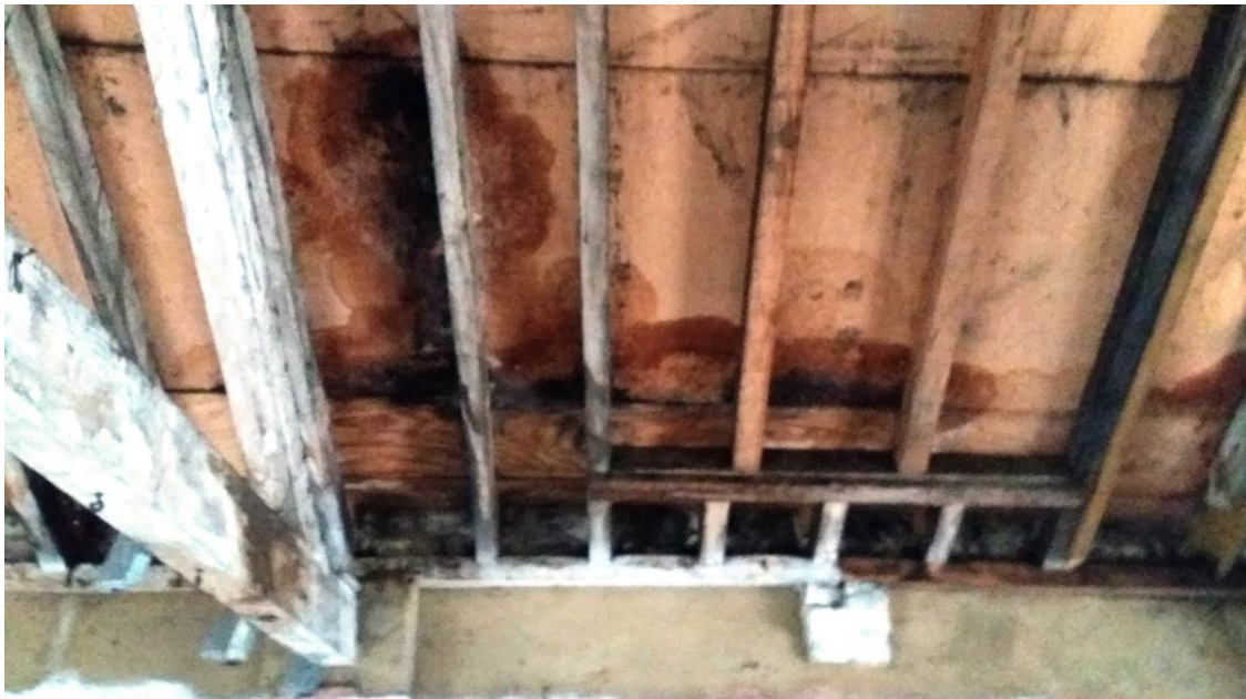
P11 - Rotting roof boards, rafters and truss end due to waterproofing failure
