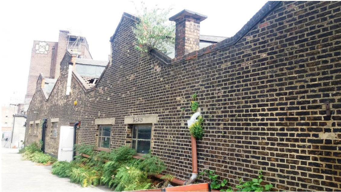
P01 – View of rear elevation showing damage to roof and lack of wall restraint
