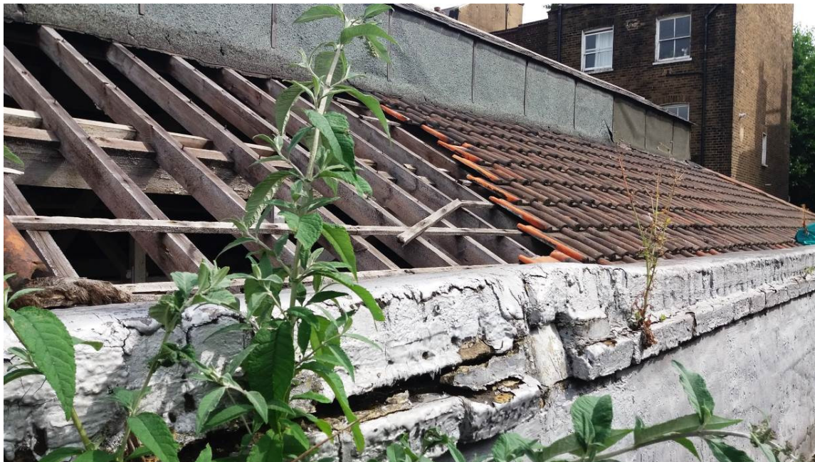
P02 – View from roof level of existing hole in roof and damage to parapet caused by vegetation growth
