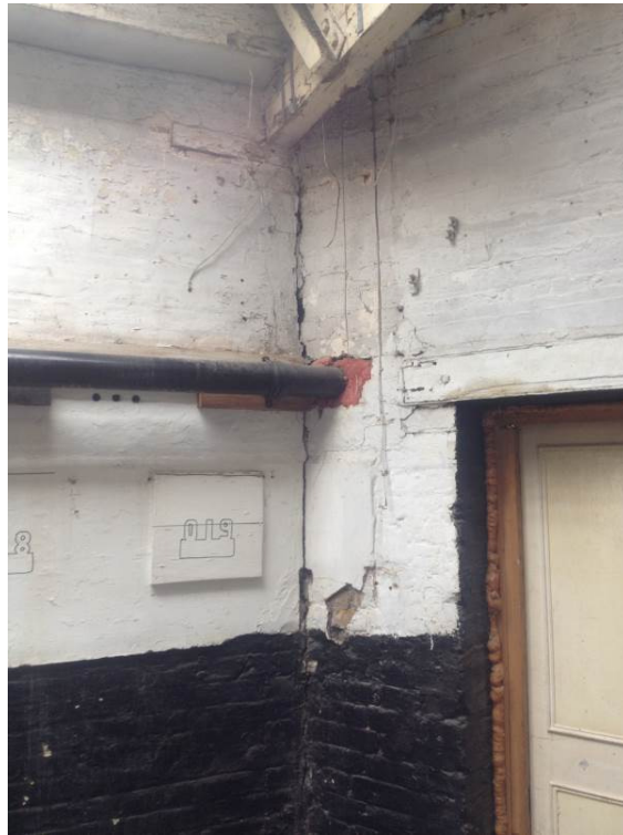
P30 – Inadequate bearing of existing roof truss.
