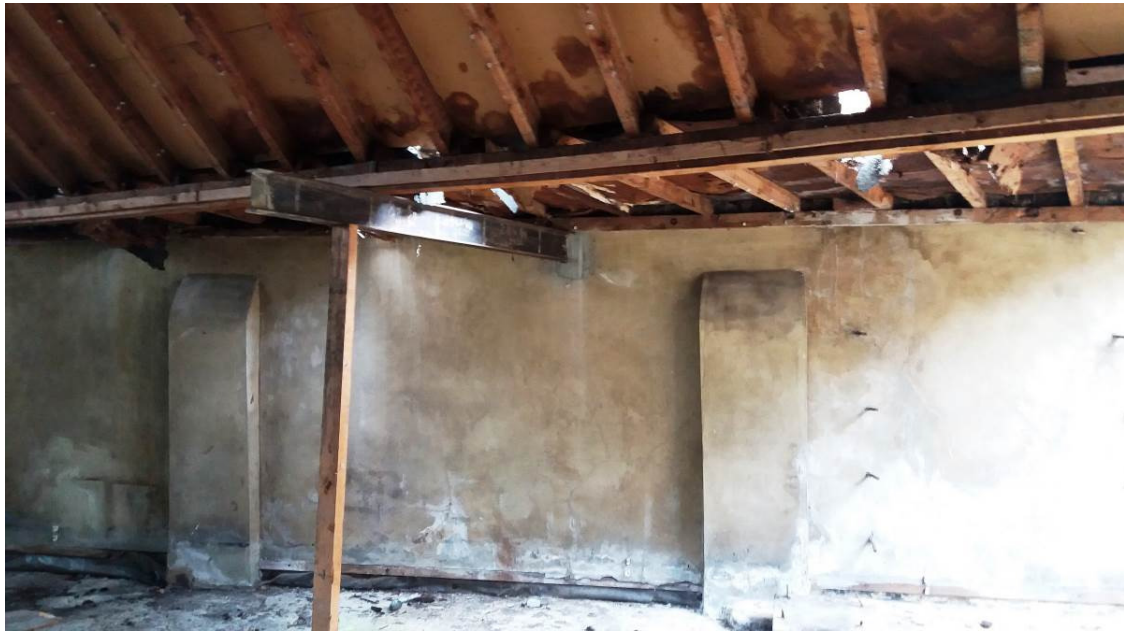
P08 – Failure of roof purlin support beam & failure of waterproofing to roof
