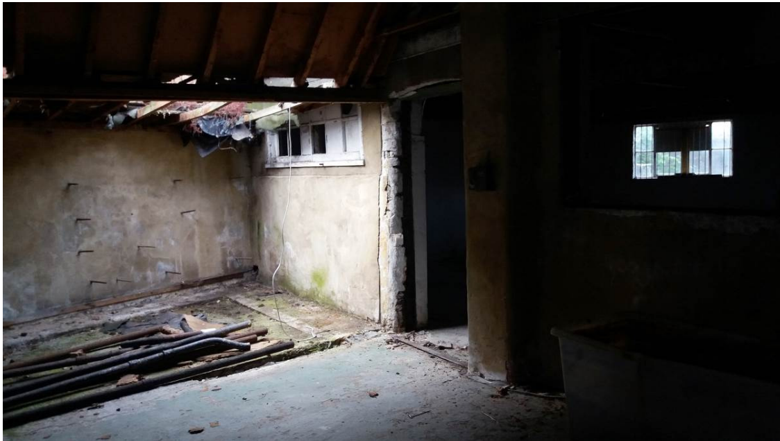
P06 – Failure of roof rafters & collapse of roof
