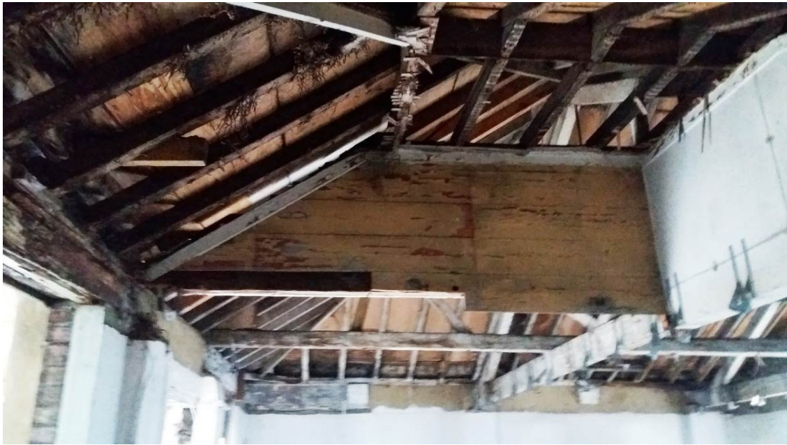
P20 – Internal vegetation on rafters caused by water ingress and wet rot to roof boards, rafters, and supporting timber beam
