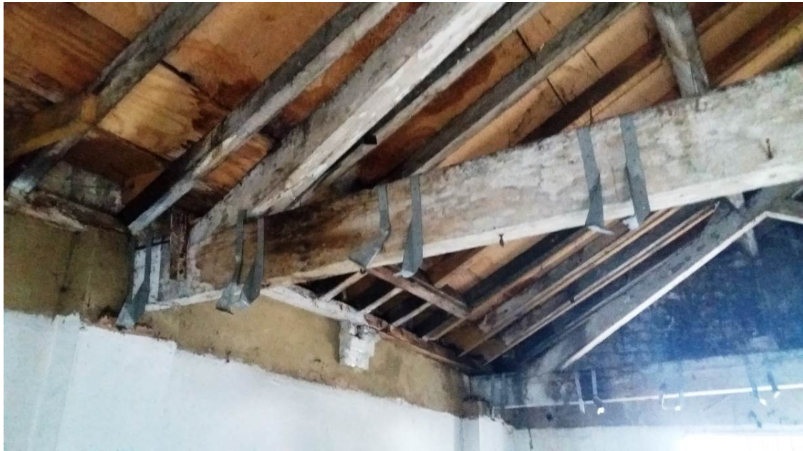
Photo 16 – Rotting roof boards, rafters, wall plate and trusses due to water ingress
