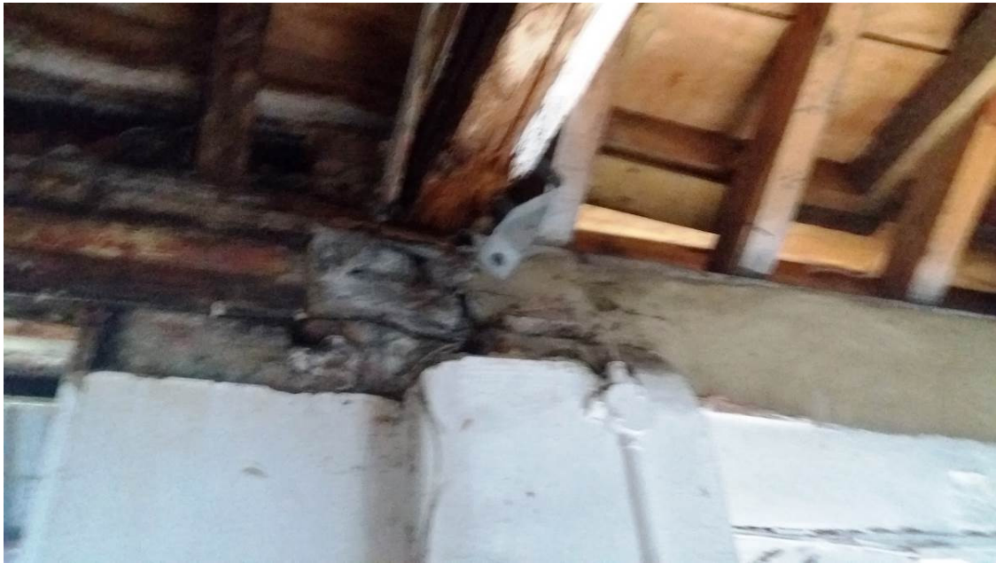
P14 – Rotting of roof structure at bearing point
