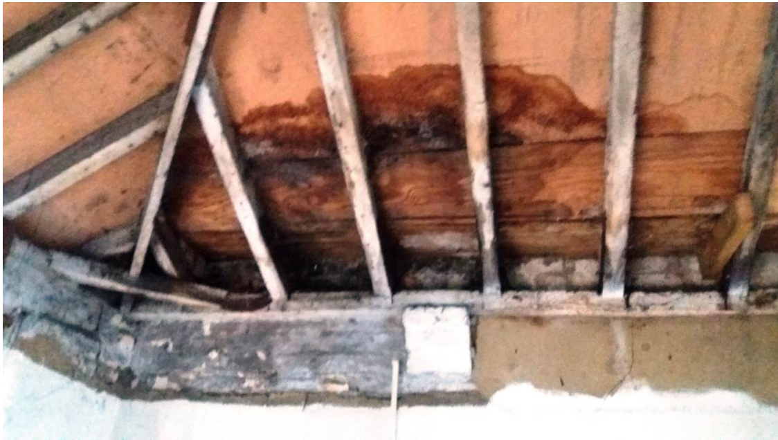
P10 – Rotting roof boards and rafters due to waterproofing failure
