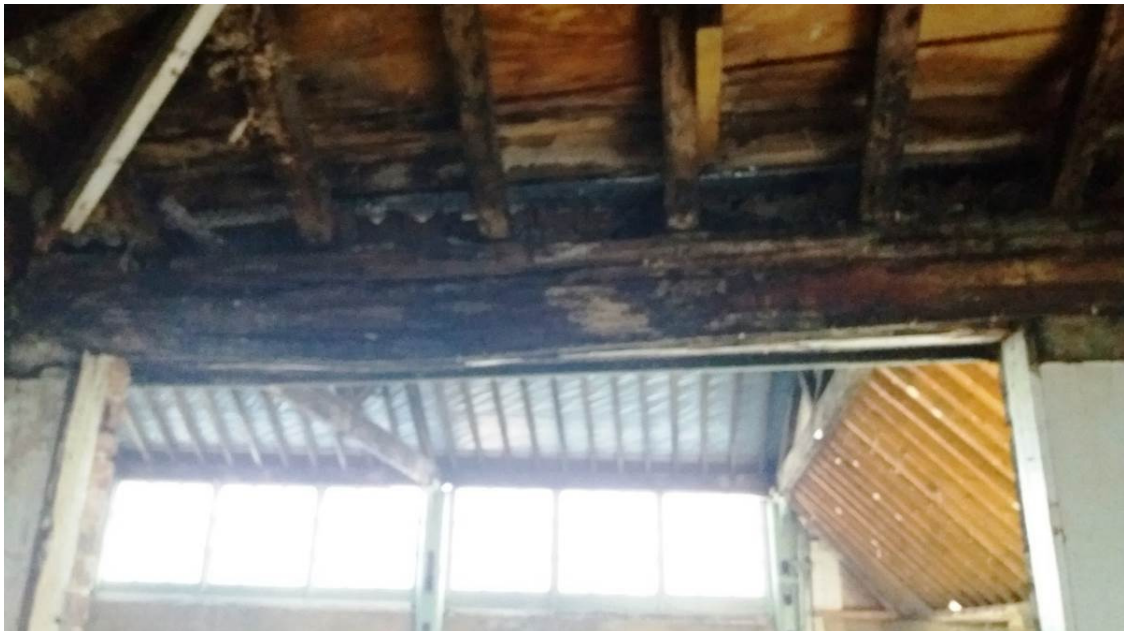
Photo 15 – Rotting roof boards, rafters and timber support due to water ingress
