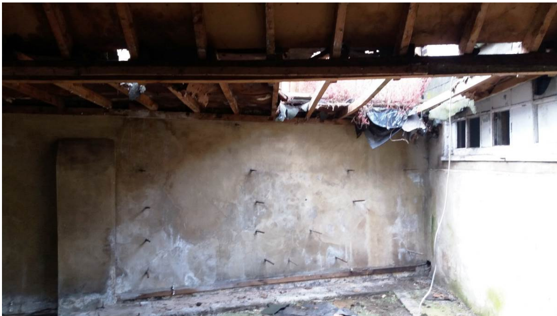
P07 – Failure of roof rafters & collapse of roof
