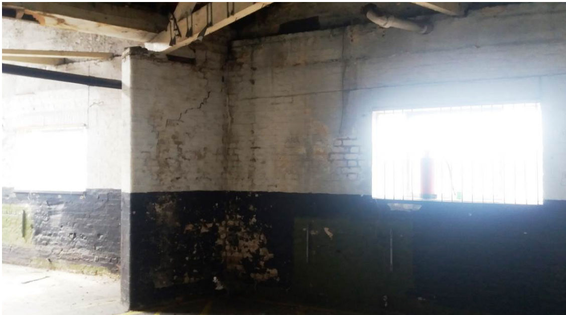
P25 – Inadequate bearing of existing roof truss.
