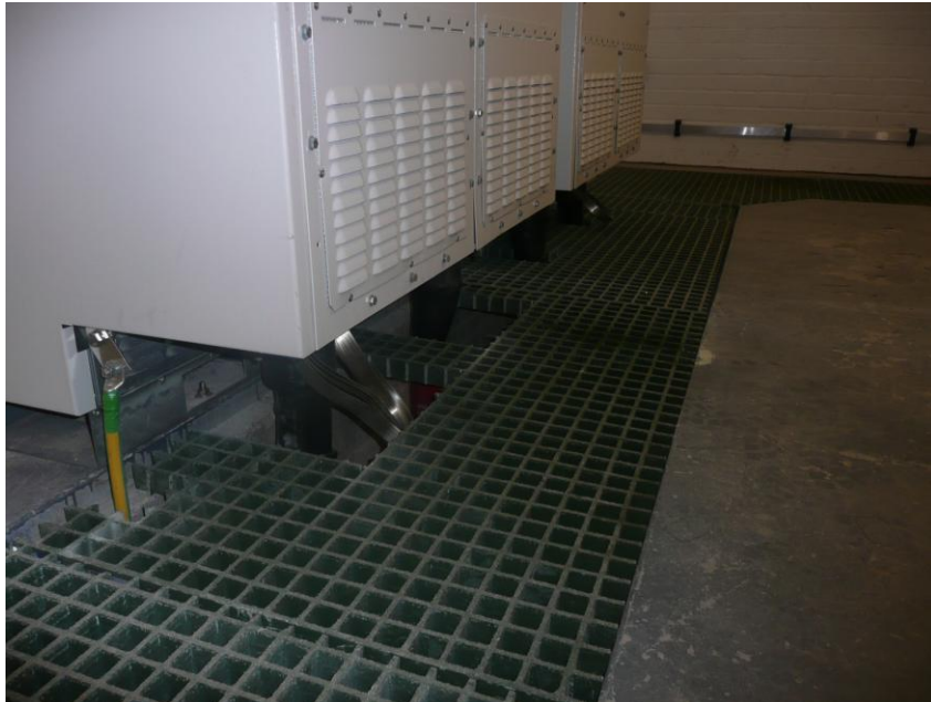
Photo 8: Example of 'cable cut-outs' in GRP grating;
