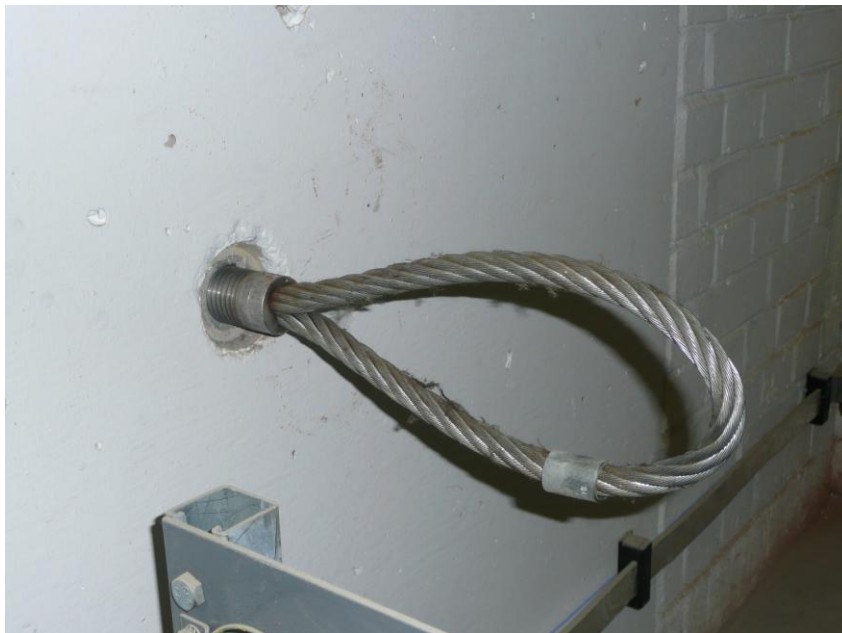
Photo 6: 'Winching eye' for plant installation ~ Example 2;
