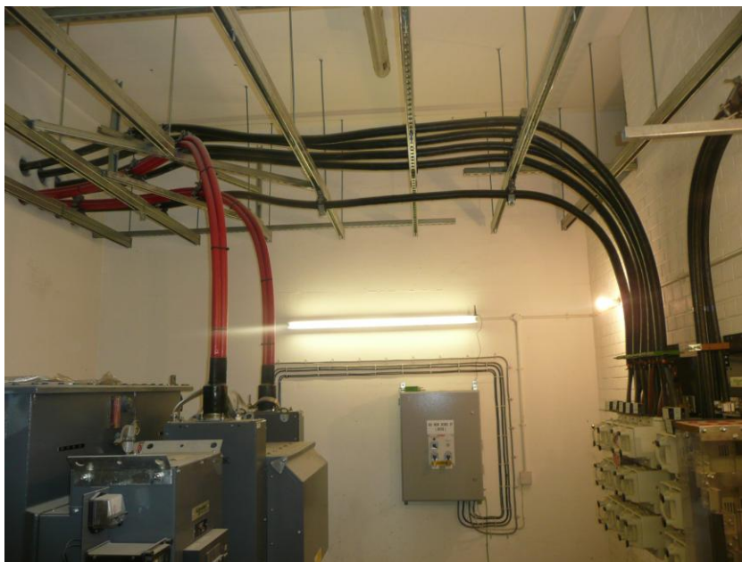
Photo 11: Example of Unistrut 'P1001T' cable supports, allowing cables to be cleated above & below;
