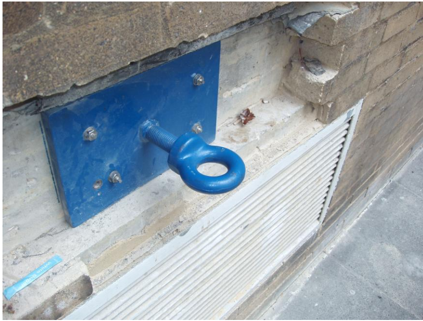
Photo 5: 'Winching eye' for plant installation ~ Example 1;
