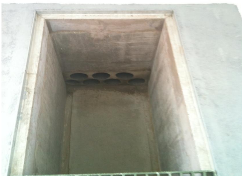
Photo 12: Example of ducts finished flush with the internal face of the substation;
